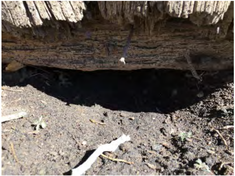
Picture 36 – The floor structure system is indeterminable. It is assumed to be sitting on wood girders with rough-sawn floor joists, which is typical for the era and similar to the exterior wall framing. The lower sections of the siding are showing decay.
