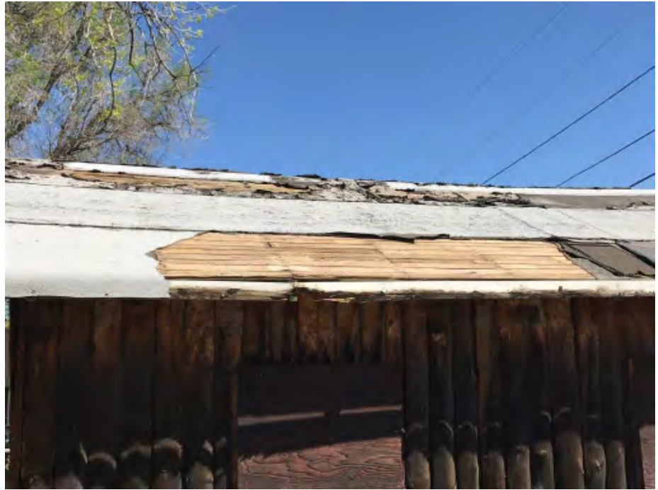
Picture 17 – Roof covering on Cabin 801, in very poor condition, urgently needs to be replaced.
