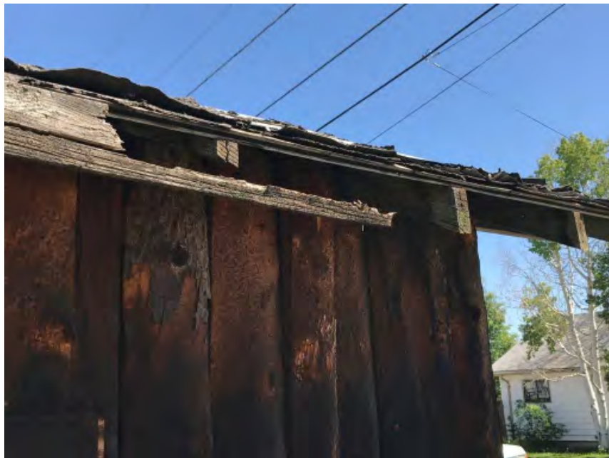
Picture 16 – Trim fascia boards on Cabin 801, note condition of trim fascia board is in decayed poor condition. If cabins are to be preserved, all roof trim boards will need to be replaced, along with new roof covering.
