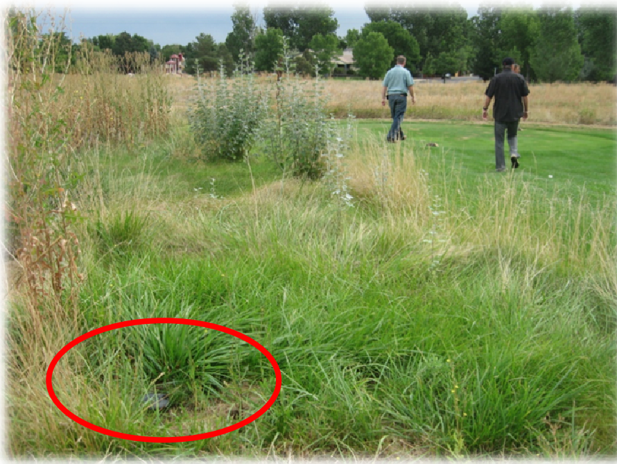
Sprinkler head outside of the formal grass limits, impacts sprinkler performance, wastes water
