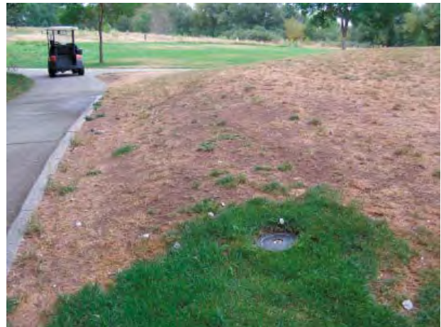
Broken irrigation head.
