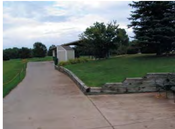
Timber retaining walls are dated & require maintenance.
