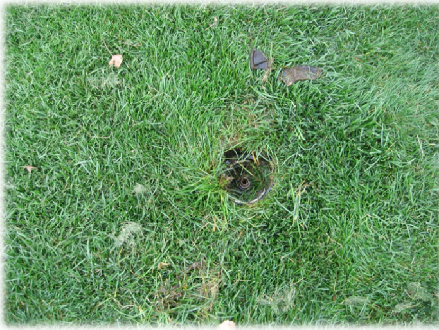
Broken head needs to be repaired
