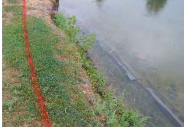
Compromised pond liner on hole 11.
