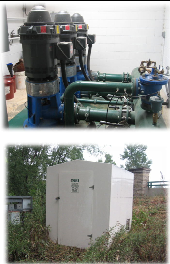
Picture 10 & 11 Main pump station & booster station building
