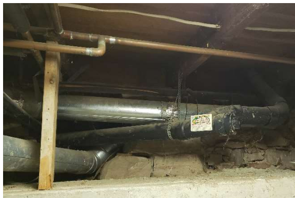
Water supply & waste lines in crawlspace
