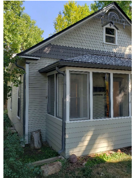
Minimal difference between top of grade and top of foundation at west side of house
