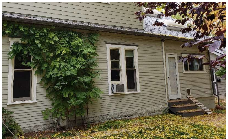
Exposed foundation increases moving east, but finish materials are in contact with grade in the southeast corner, around the now-enclosed deck
