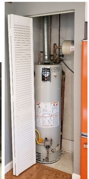
Water heater in kitchen
