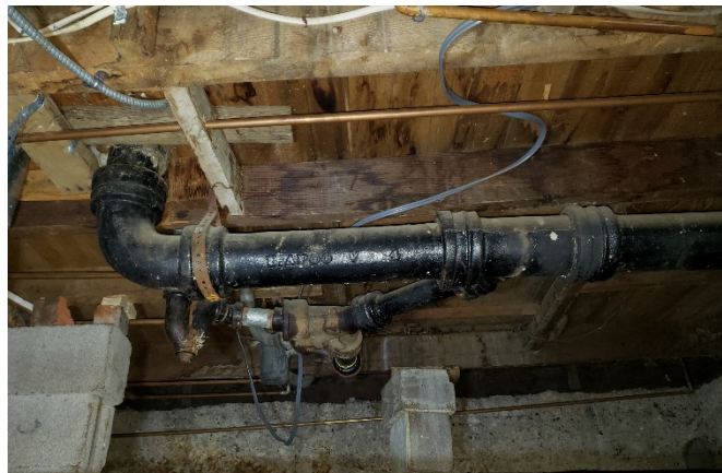
Copper water supply and cast-iron waste lines.
