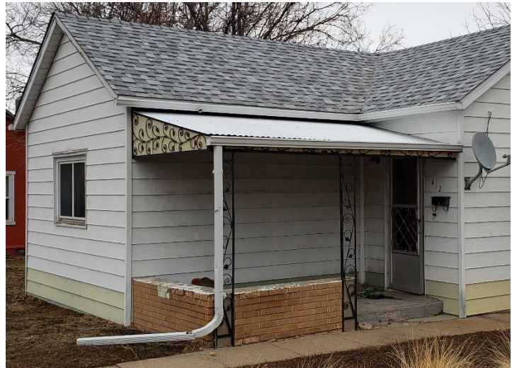
Upper roof gutters discharge water directly onto covered porch roof.
