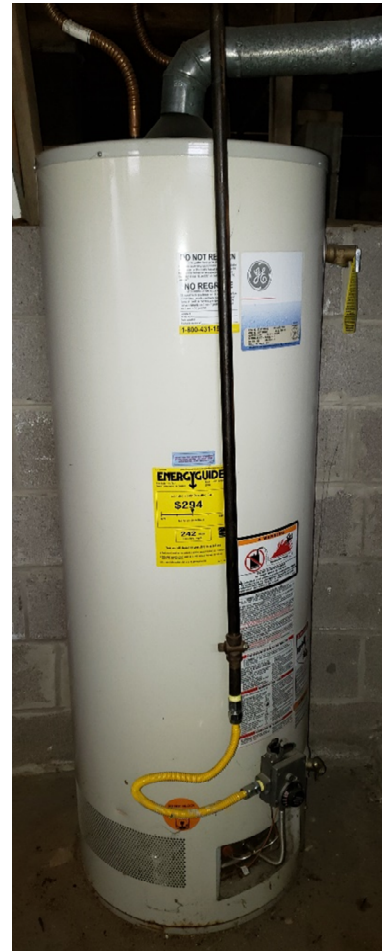
40-gallon gas-fired water heater.
