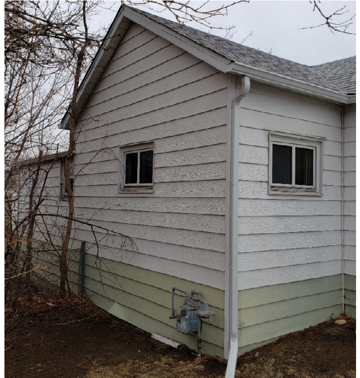
Aluminum siding. One panel is bent near grade on the north side and the siding has been damaged around the west facing window where an awning was removed.
