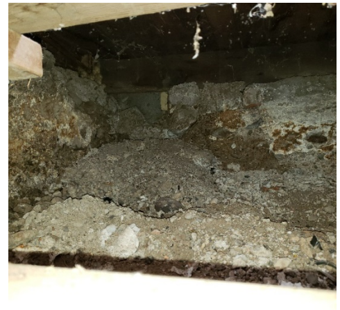
Failing foundation wall in southeast corner of house.
