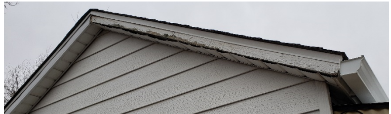
Missing fascia & sagging soffit at west gable end. Original barge rafter exposed.
