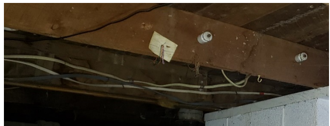
New romex wiring with abandoned knob-and-tube.
