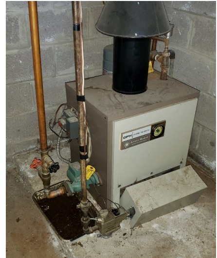
Gas-fired boiler located in basement.
