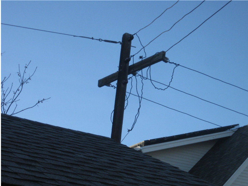
Figure 31. 109 W. Spruce old wiring on north end of garage, facing northwest.
