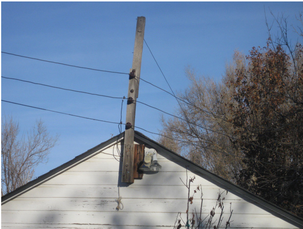
Figure 32. 109 W. Spruce old wiring on west end of shed 3, facing east.
