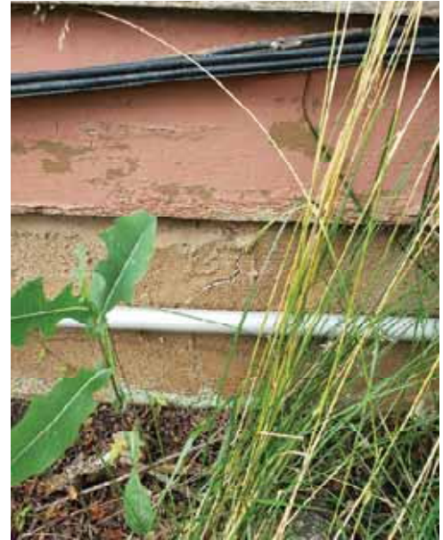
Foundation cracking viewed from the exterior.
