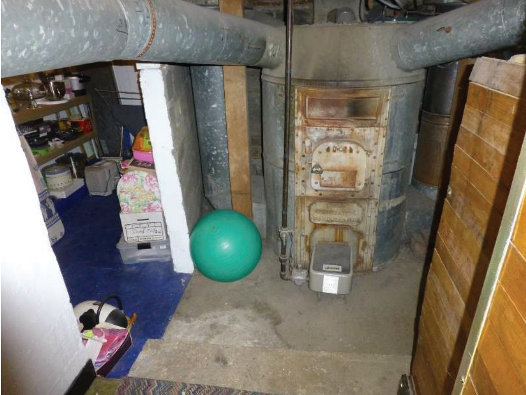
Converted coal furnace
