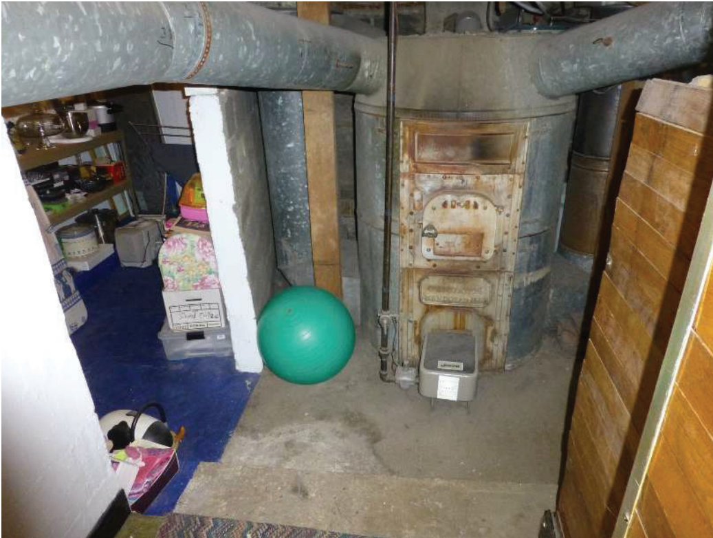
Converted coal furnace
