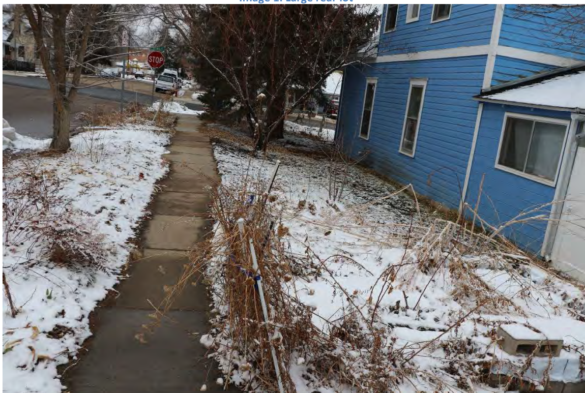
Image 2: Grading. Drainage slopes towards the house on the west elevation
