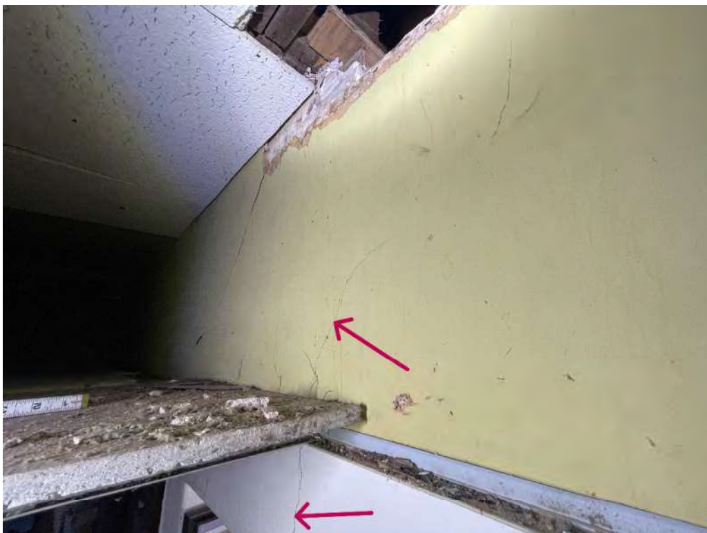
Figure 4: Crack at header between original house and addition
