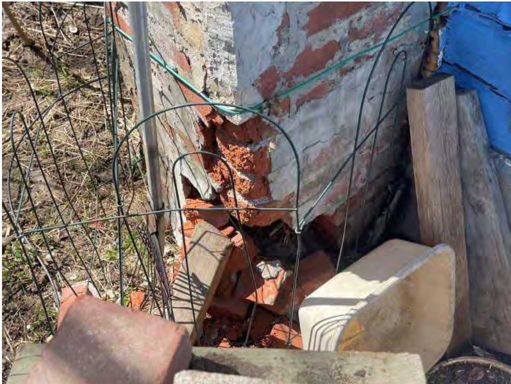
Figure 3: Missing bricks at base of chimney along east elevation
