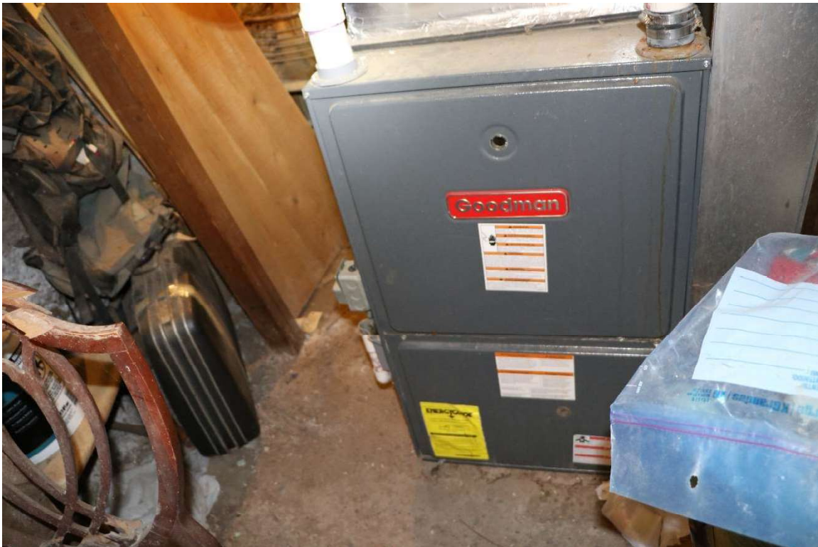
Image 37: Heating and Air Conditioning. Furnace
