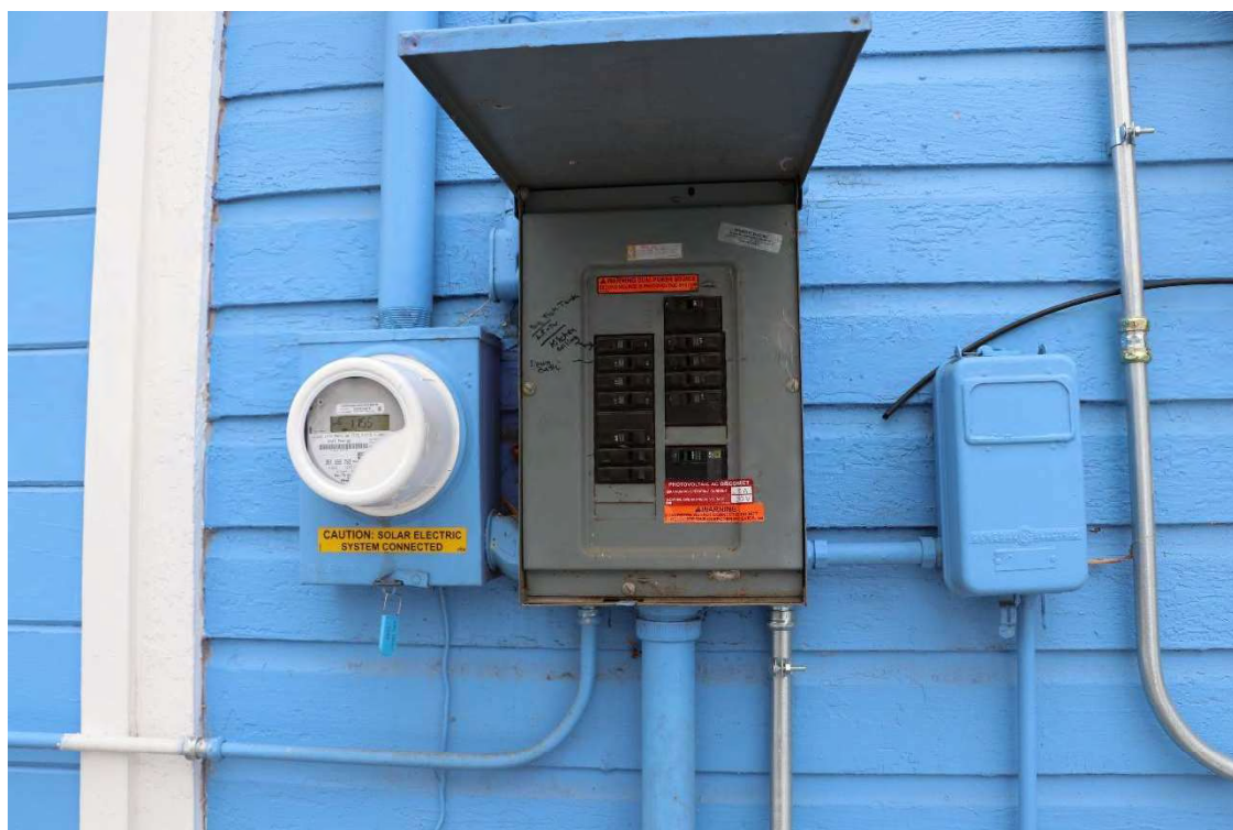
Image 41: Electrical Service and Panels
