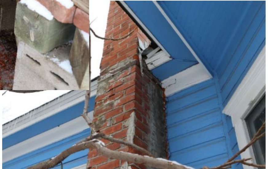
Photos of the chimney in disrepair from the 2024 HSA.
