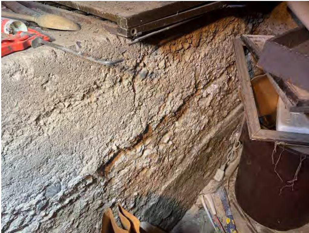
Figure 9: Inside face of concrete retaining wall. Note loss of cement paste and exposed aggregate due to moisture migration
