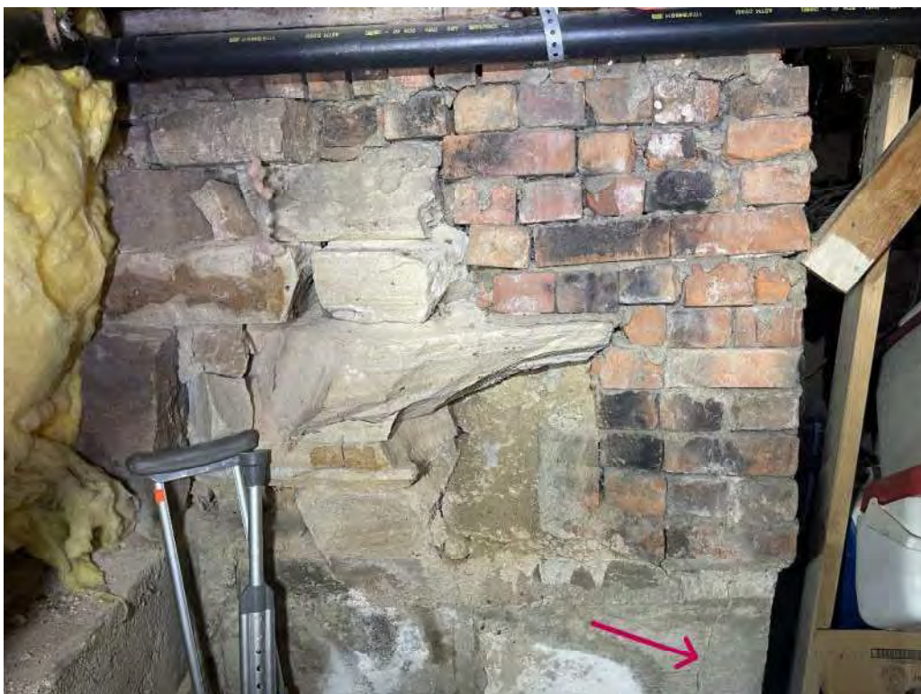
Figure 10: Area of foundation wall at stone to brick interface due for partial reconstruction
