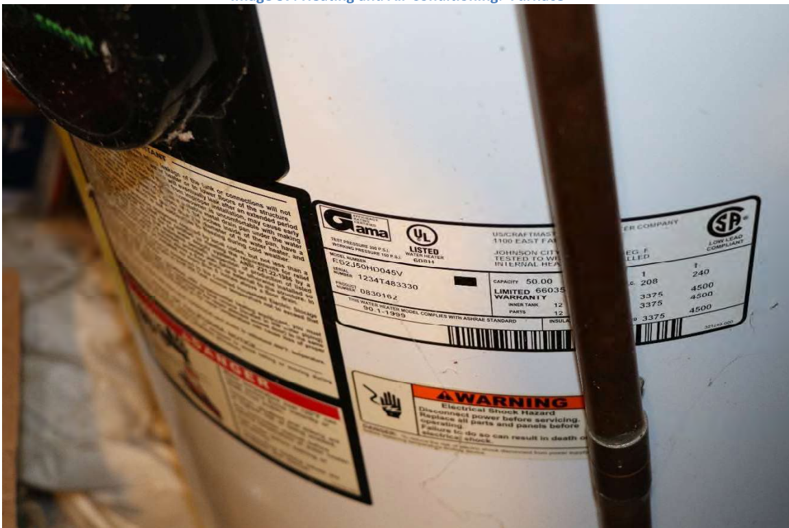
Image 38: Heating and Air Conditioning. Hot water heater
