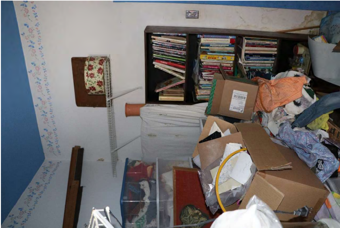
Image 28: Wall finishes. First floor. Typical conditions. Note the water stain by the door casing
