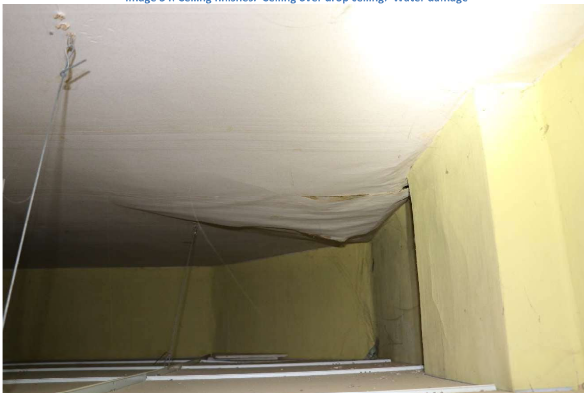
Image 35: Ceiling finishes. Ceiling over drop ceiling. Water damage
