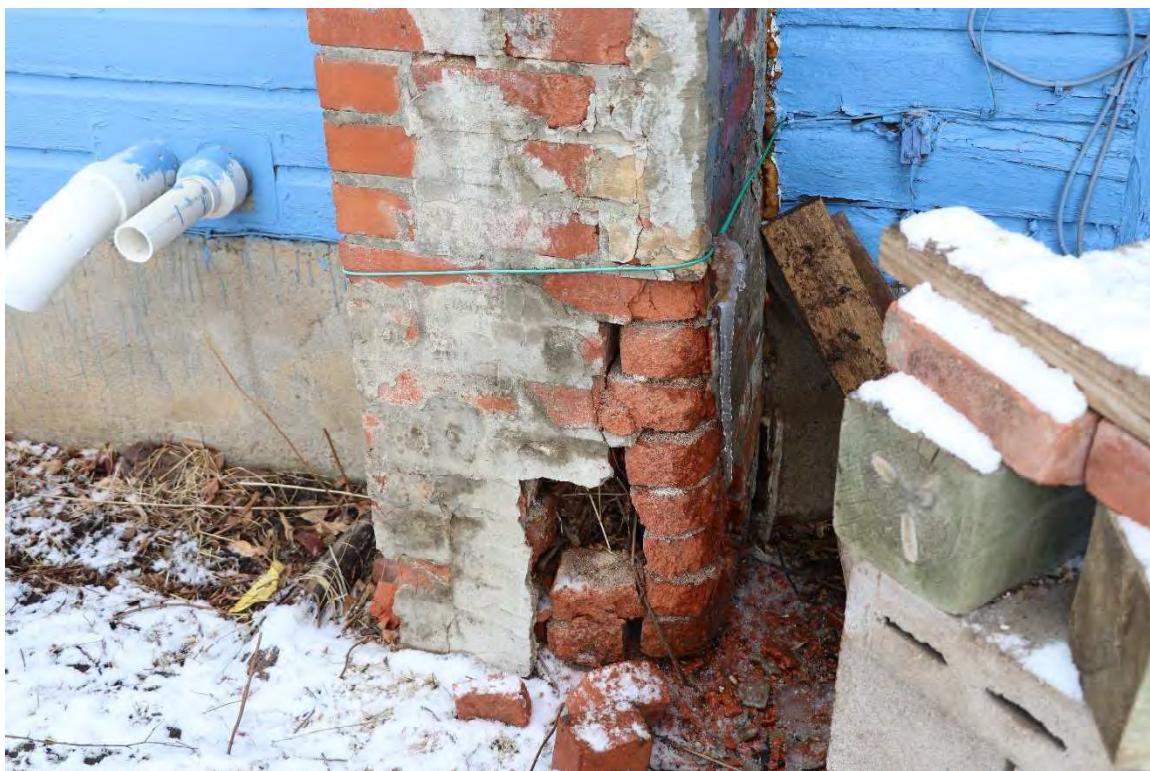
Image 15: Brick chimney base. Advanced deterioration from moisture
