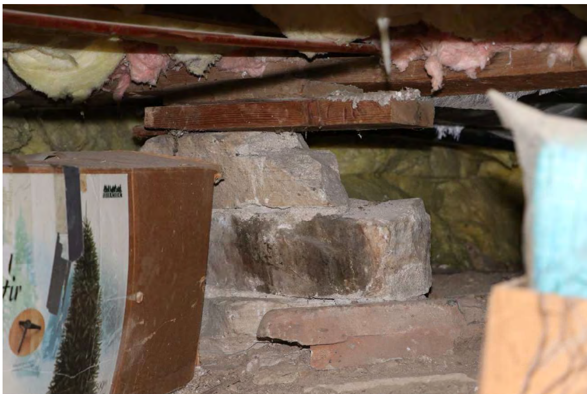
Image 6: Stacked stone partial-span pillar. Note the added wood boards above and the minimal bearing surface
