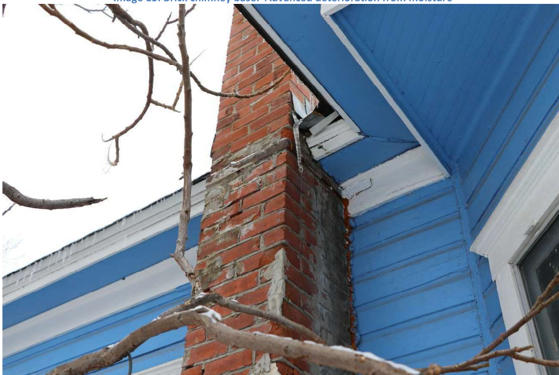
Image 16: Water from the roof drains directly onto the chimney
