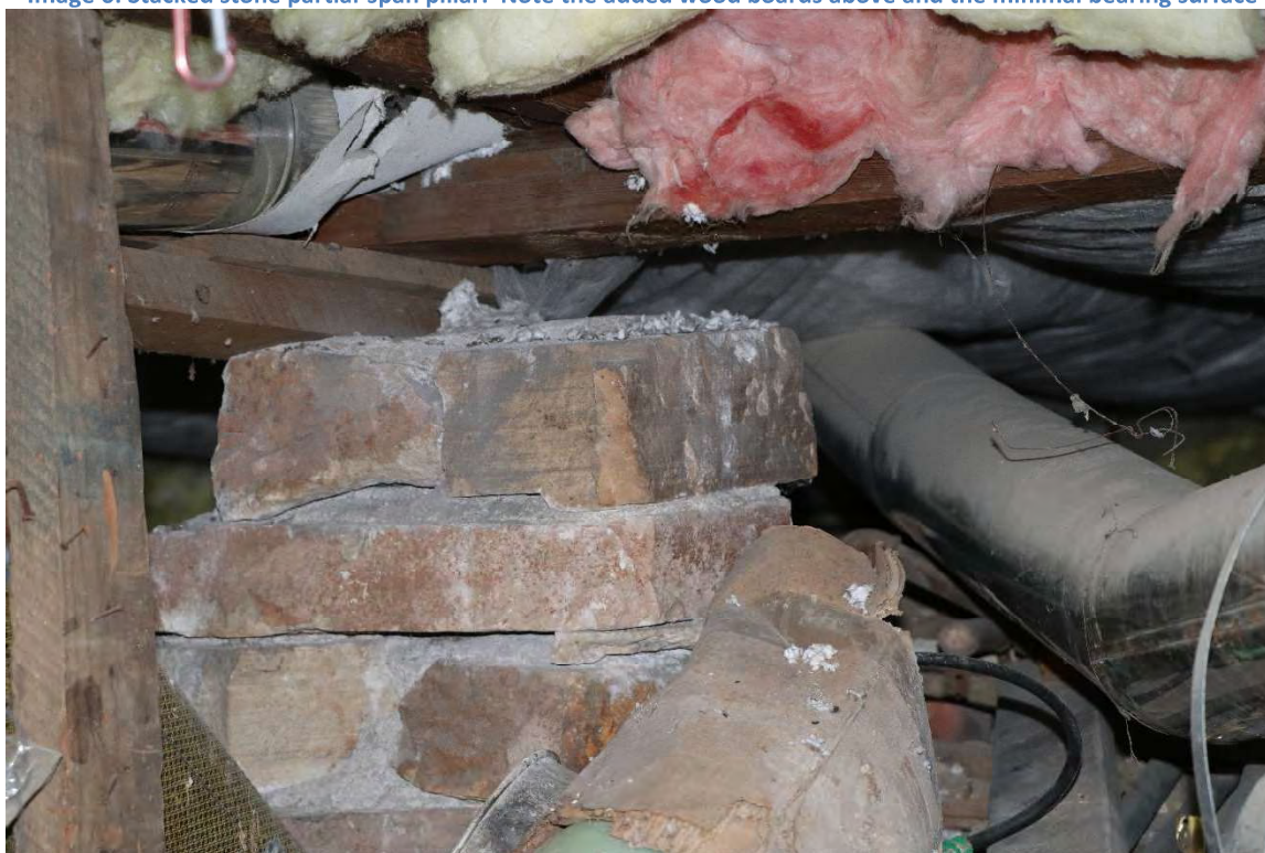
Image 7: Stacked stone pillar. No longer providing support
