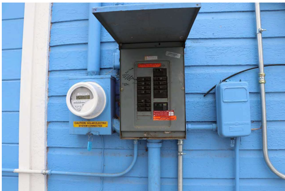
Image 41: Electrical Service and Panels
