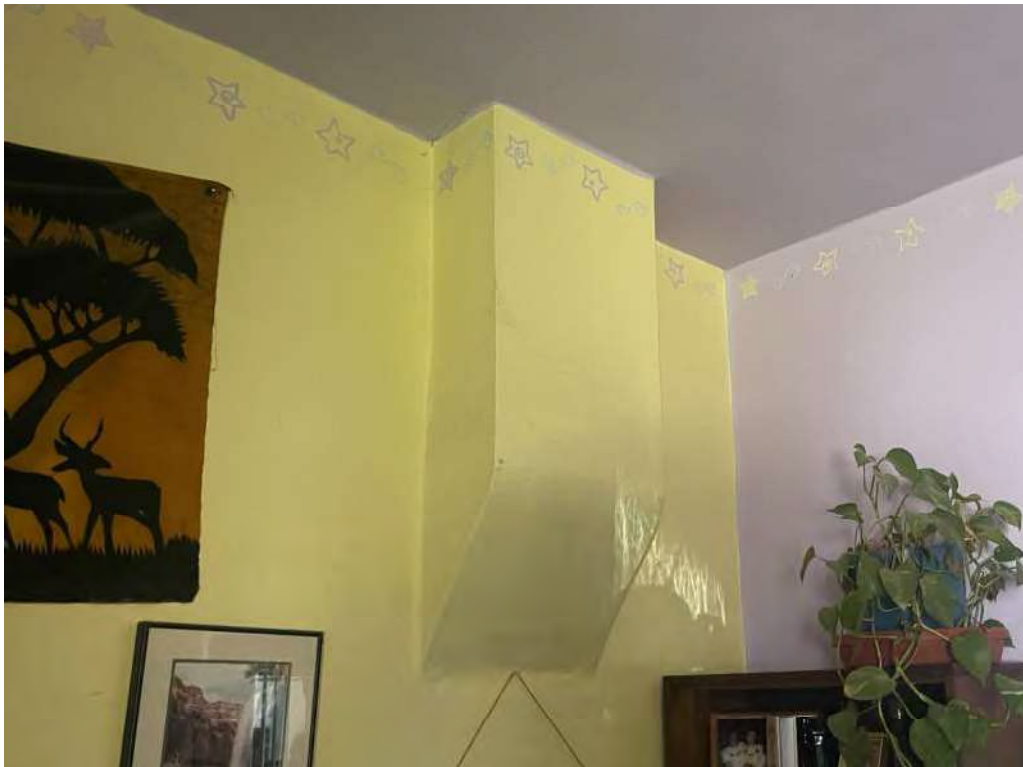
Figure 2: Interior chimney corbel at partition wall
