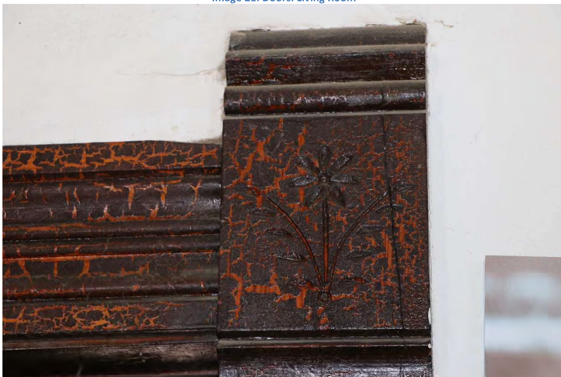
Image 22: Doors. Living room. Shellac deterioration detail
