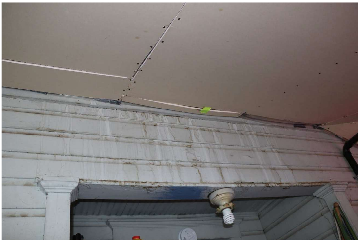
Image 13: South elevation. Note the water staining from water infiltration at the enclosed porch roof /wall junction
