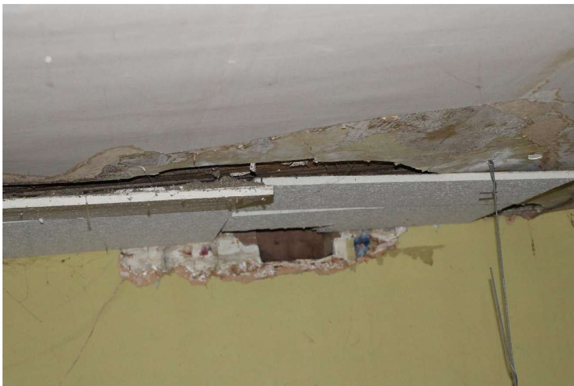
Image 34: Ceiling finishes. Ceiling over drop ceiling. Water damage
