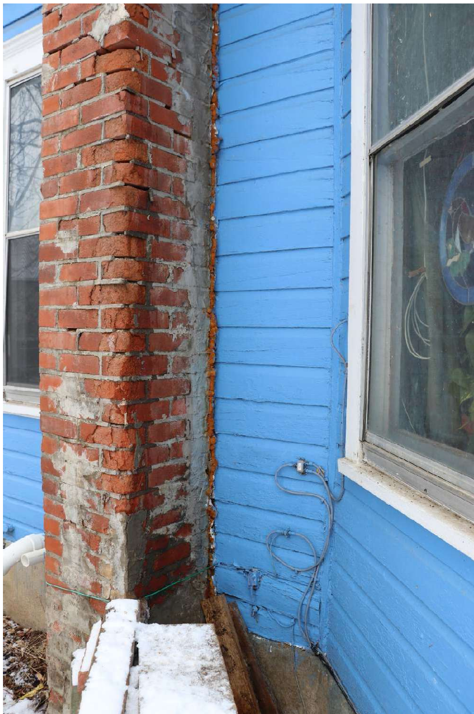
Image 17: Deterioration is evident along the length of the chimney below the roofline
