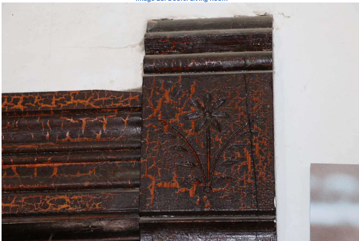
Image 22: Doors. Living room. Shellac deterioration detail
