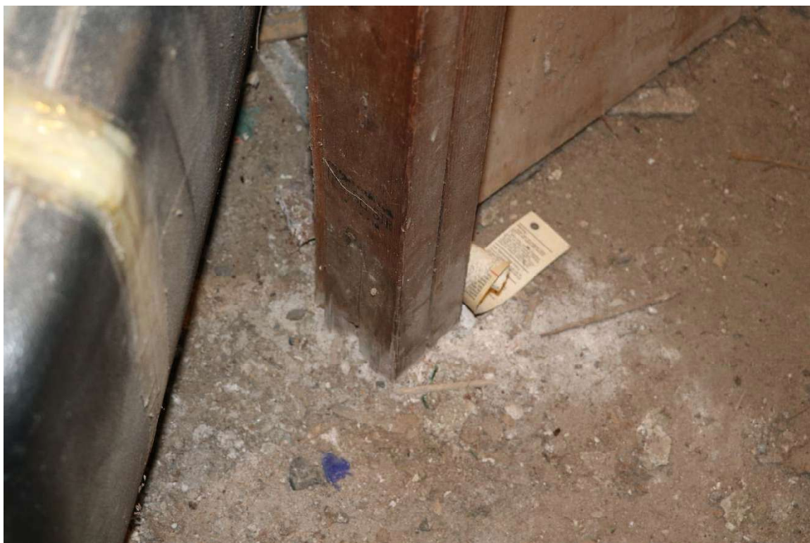
Image 8: Joist support beam. Set directly on the dirt floor
