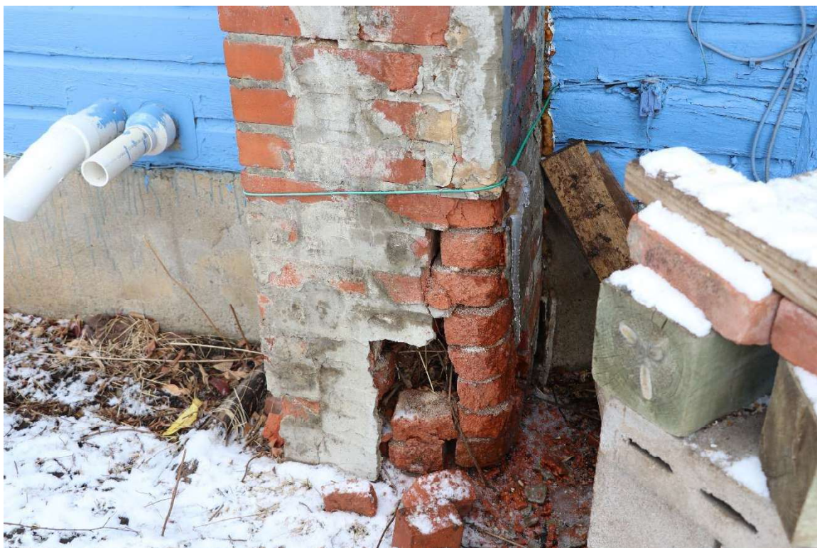
Image 15: Brick chimney base. Advanced deterioration from moisture
