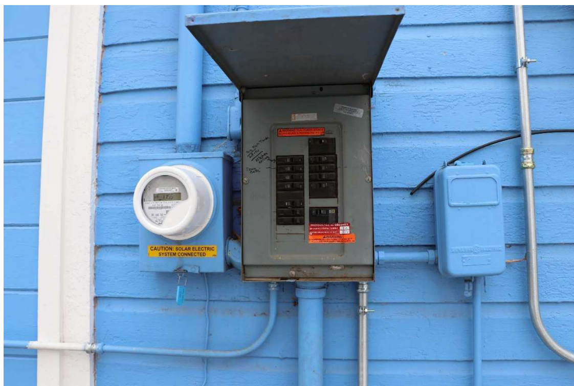
Image 41: Electrical Service and Panels
