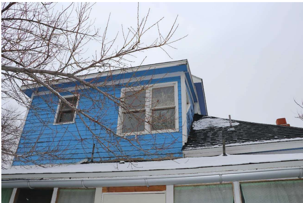
Image 39: Ventilation. Plumbing vents
