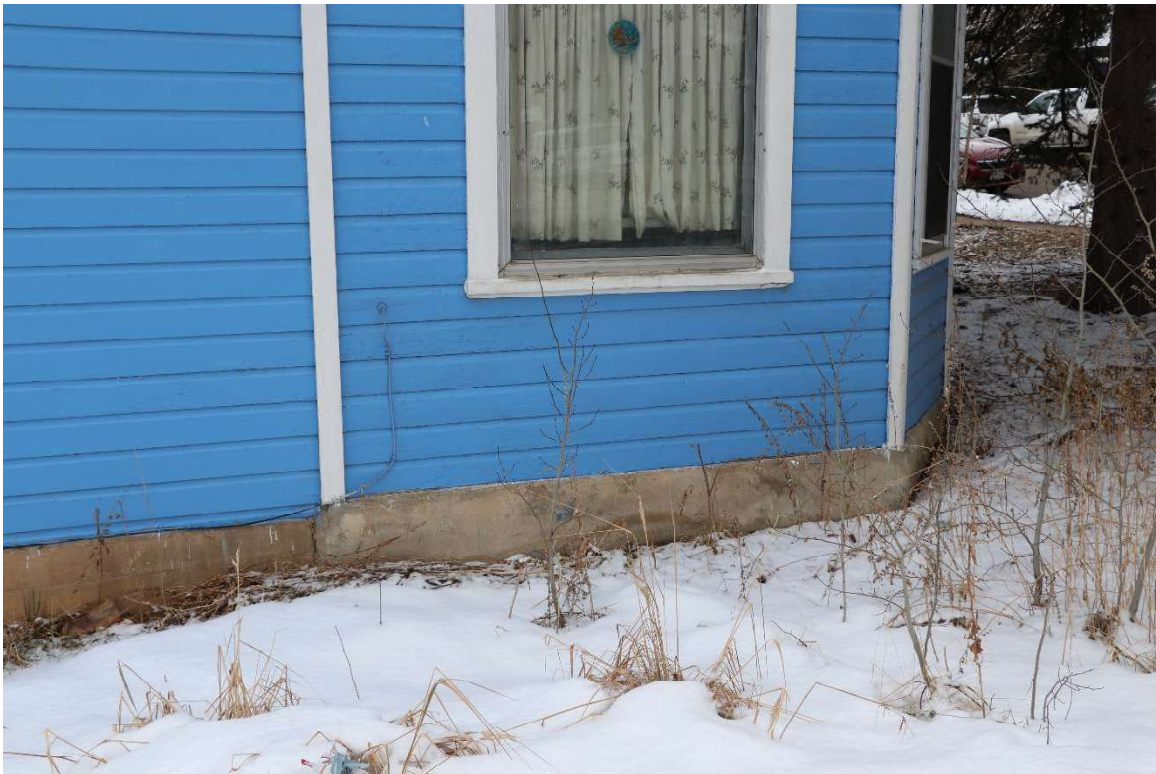
Image 5: Foundation. Seam visible under the addition on the left of the image
