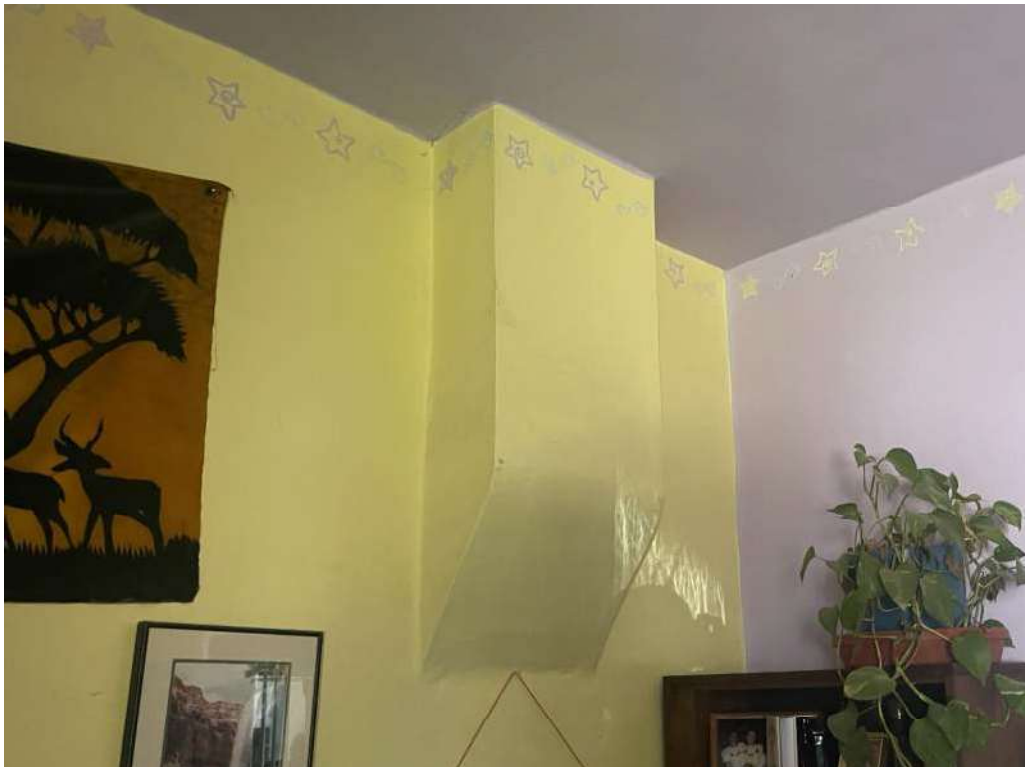
Figure 2: Interior chimney corbel at partition wall
