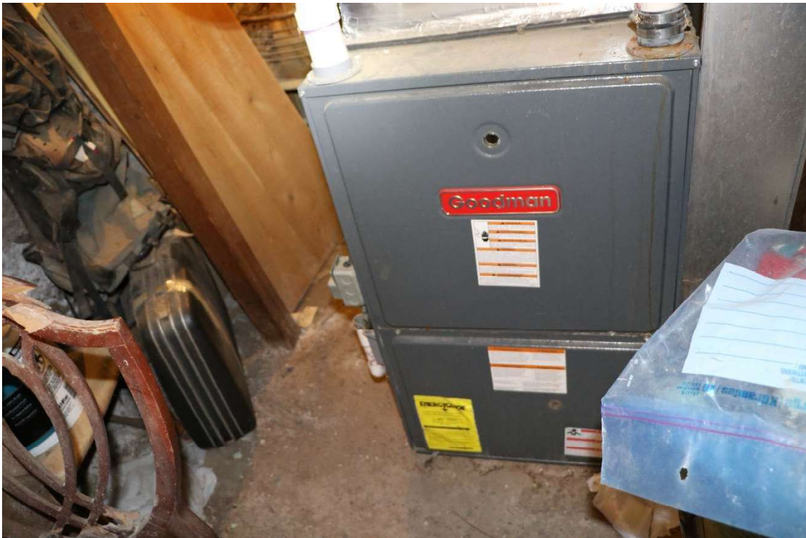
Image 37: Heating and Air Conditioning. Furnace
