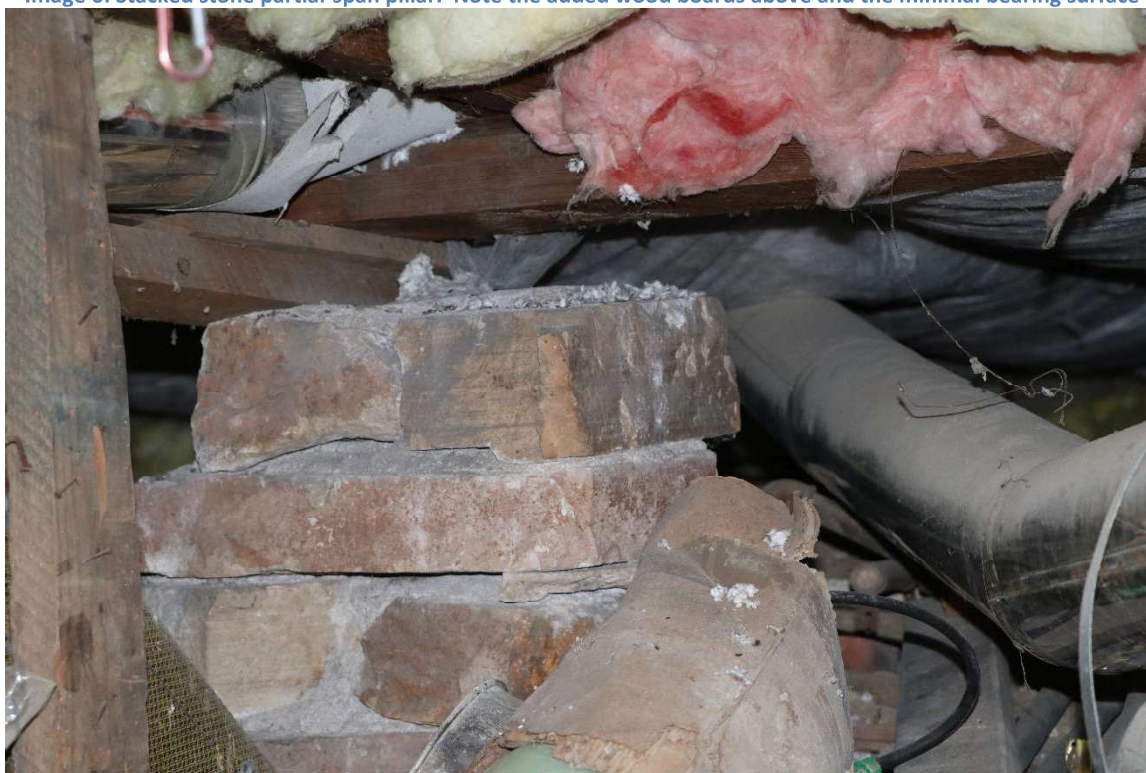
Image 7: Stacked stone pillar. No longer providing support
