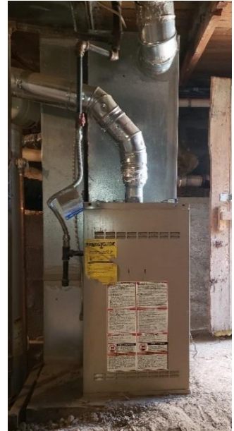
Gas furnace located in the crawlspace.
