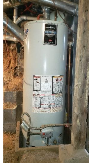
Gas water heater located in the crawlspace.
