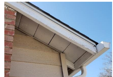
Exposed roof sheathing and rafter tails.
