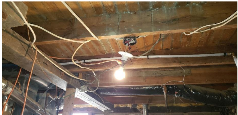
Romex wiring is seen throughout the crawlspace.
