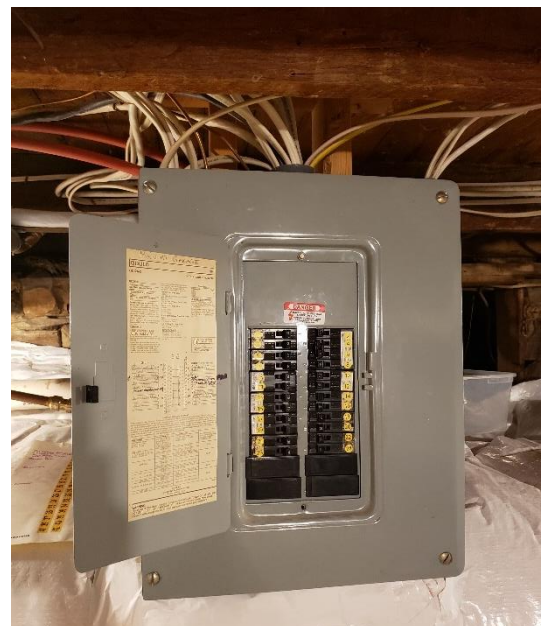
Sub-panel in the house basement.
