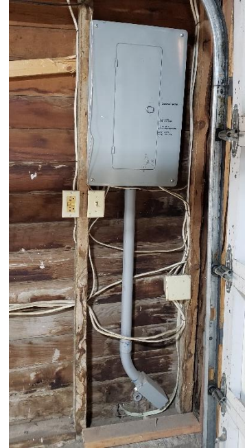
Main electrical panel in the garage.
