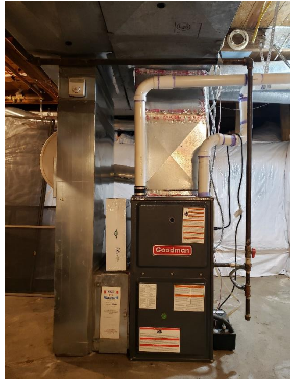
Furnace and ductwork in the basement.
