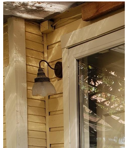
Wall sconce at the east addition.
