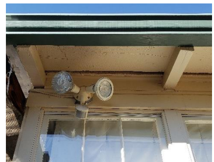
Flood light at east exterior wall.
