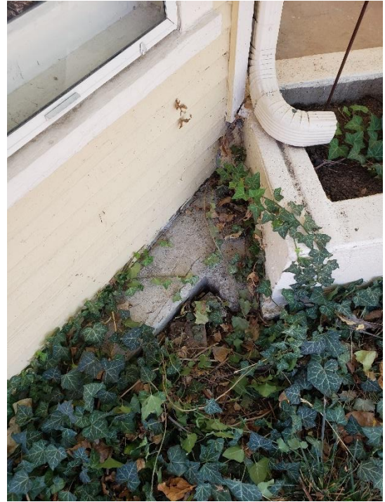
The top of grade sits at or near the top of the foundation on the west side of the house.
