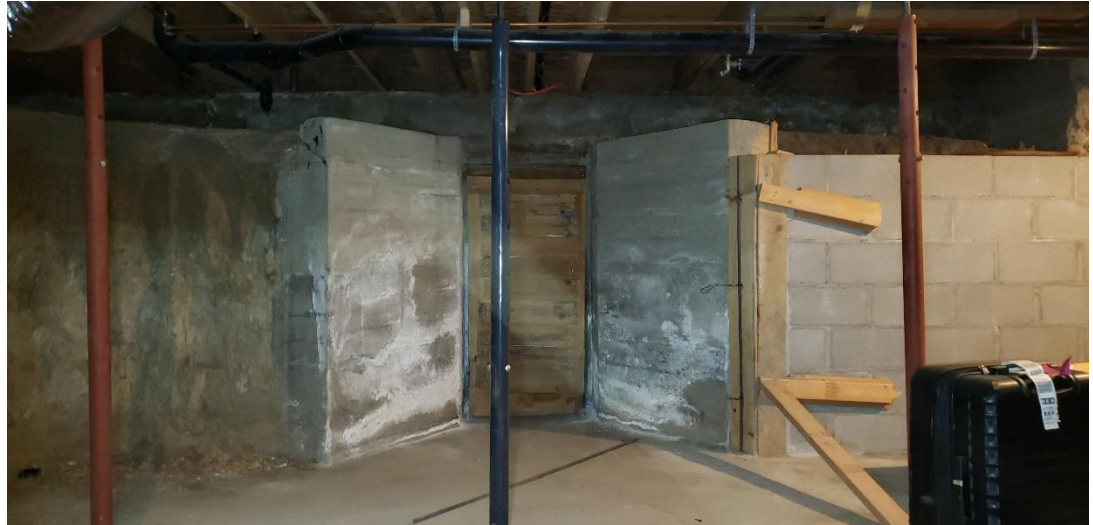
Entrance to the coal room. Unsupported grade on the left and a CMU wall intended for retaining on the right.
