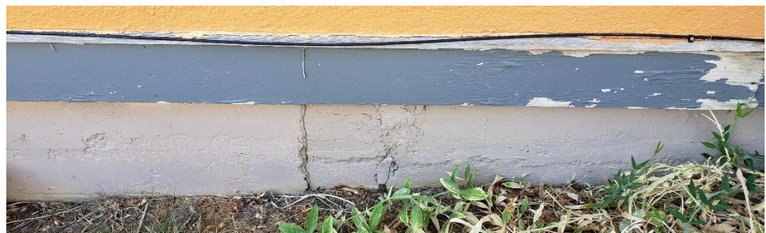
The original foundation on the right and the east addition on the left. A vertical cold joint distinguishes the two.
