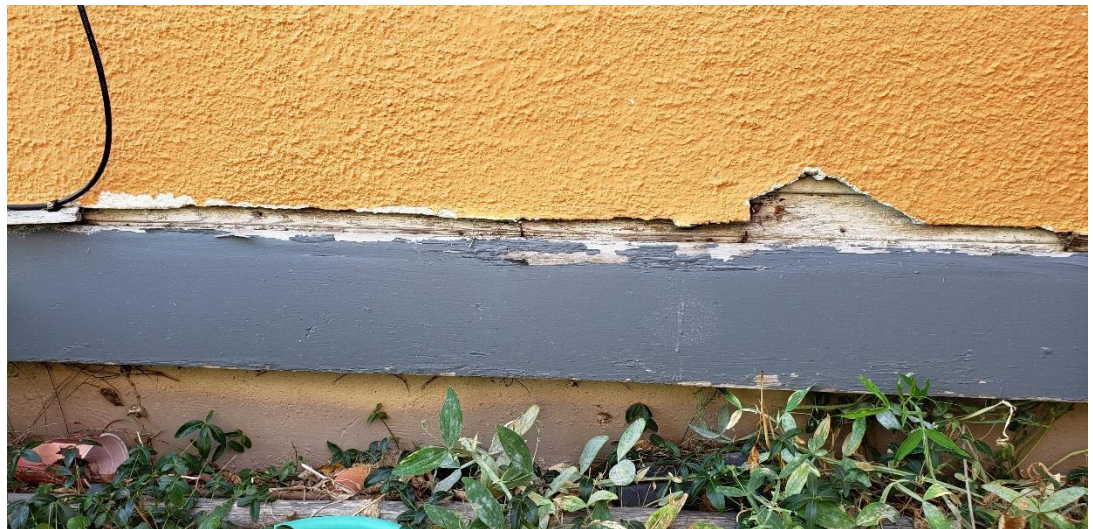
The stucco is damaged at the wall base. There appears to be wood clapboard siding beneath the stucco.
