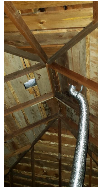
Broken ridge beam of original roof.
