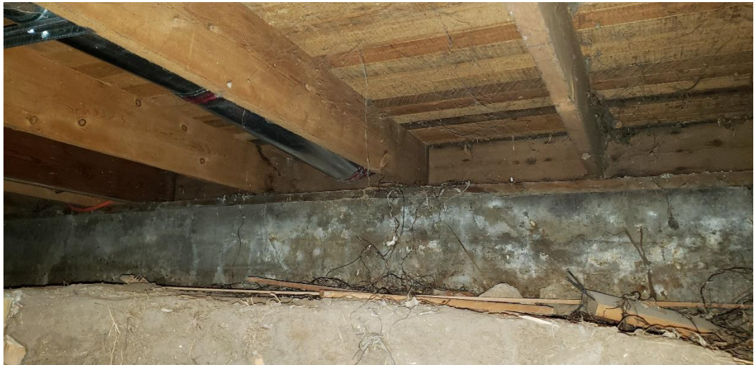
Original floor joists & sheathing. Water damage is apparent on the rim and sill plate.
