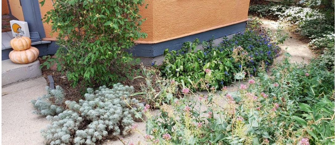
Grade sits close to finish materials at the west side of the house with minimal slope away from the foundation.
