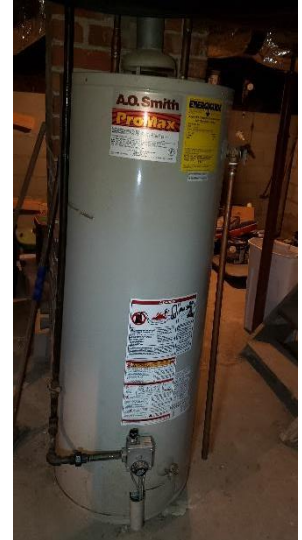
Water heater in the basement.
