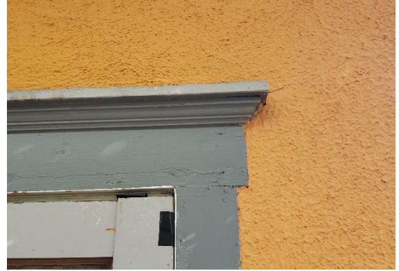
Cracked stucco is seen at several windows and doors. The door trim is nearly flush with the stucco, indicating an additional siding layer beneath the stucco.
