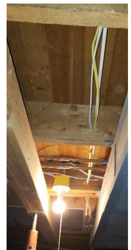
Romex wiring is seen in the basement & attic.
