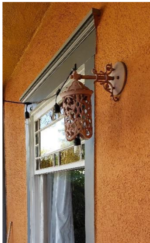
Wall sconce at front porch.
