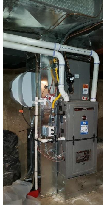
Gas furnace in the basement.
