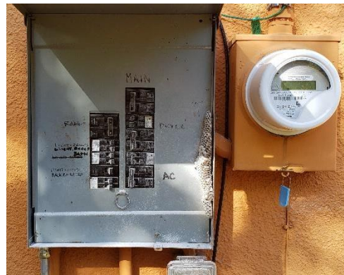
Electrical panel & meter.
