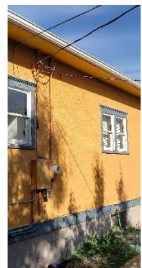
Overhead electric service to the east side of the house.
