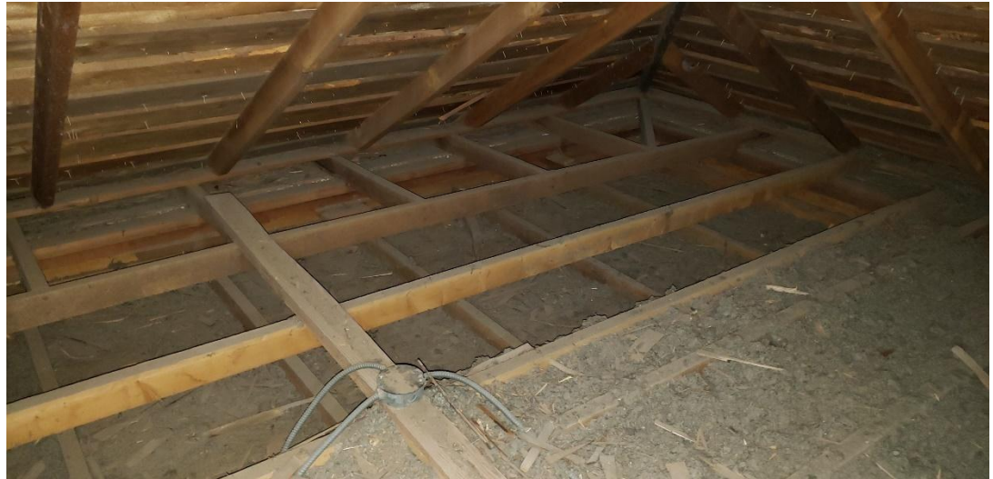
The covered front porch roof is dropped below the main roof ceiling joists.
