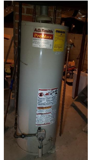
Water heater in the basement.
