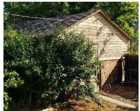
Southwest view of the garage. The roof is sagging and deteriorated.
