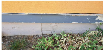
COLD JOINT SEAM IN THE CONCRETE FOUNDATION INDICATES THE EXTENT OF THE ORIGINAL HOUSE.
