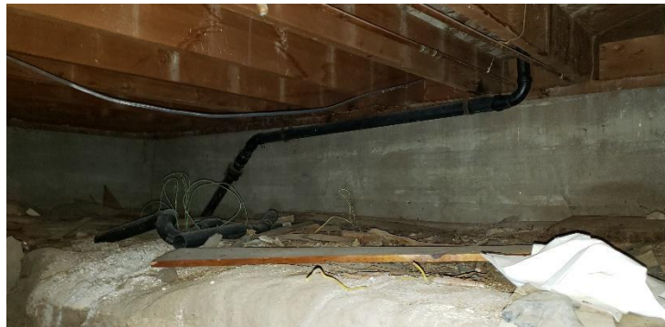
Copper water supply lines. The ABS plastic waste lines terminate at a cast iron waste line.
