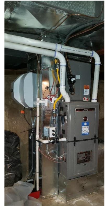
Gas furnace in the basement.
