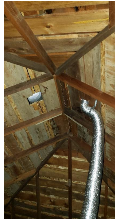
Broken ridge beam of original roof.
