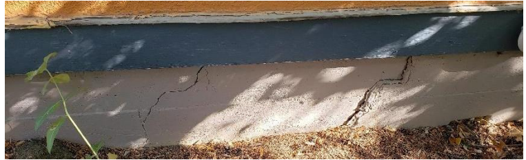
Foundation wall cracks on south side exterior.
