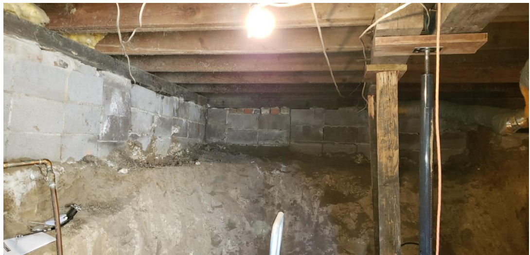
CMU foundation with various bonds, seams, grout, and heights. The excavation is unsupported.
