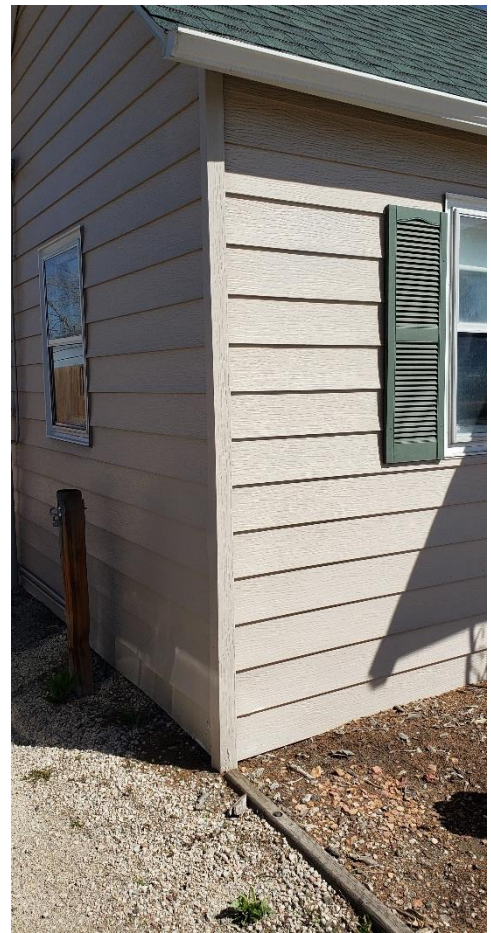
Southwest corner of the house where the siding meets grade.
