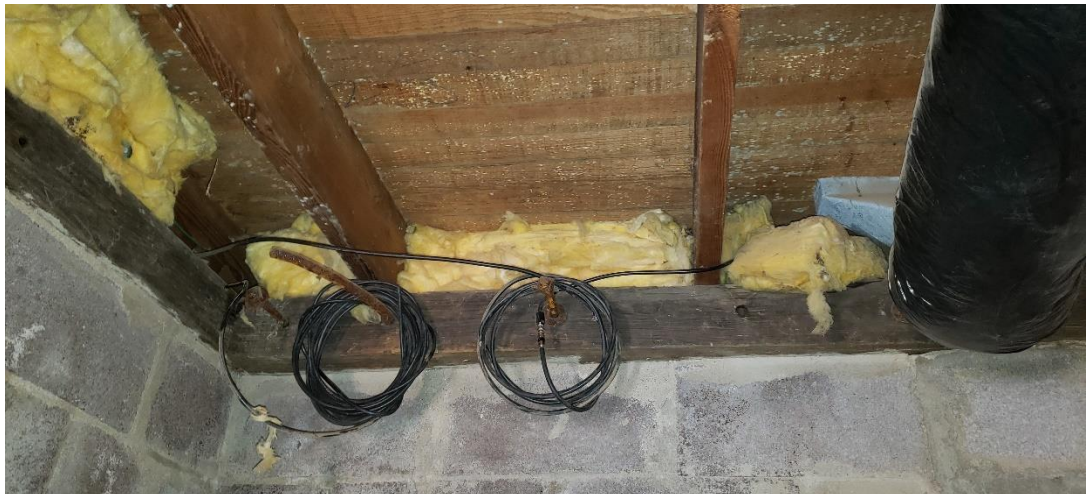
Original flooring, 2x8 floor joists, and sill plate. The sill plate appears to be taken from a boxcar frame.
