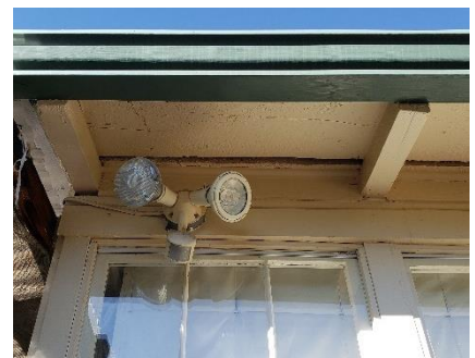
Flood light at east exterior wall.
