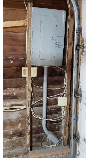
Main electrical panel in the garage.
