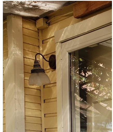
Wall sconce at the east addition.
