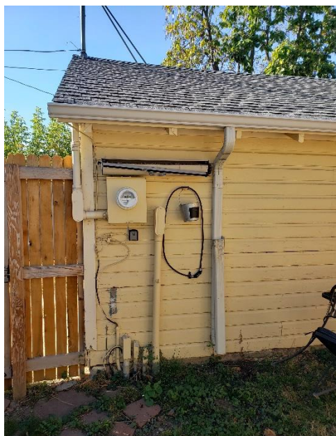
Electrical meter on the north side of the garage.
