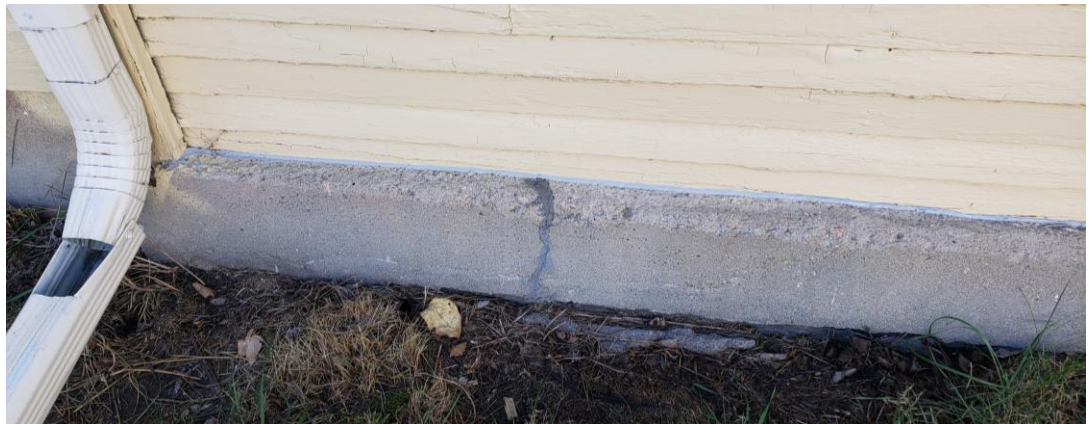
The concrete face over the stone foundation is cracked and does not extend below grade in most areas.
