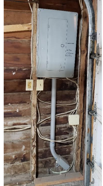
Main electrical panel in the garage.
