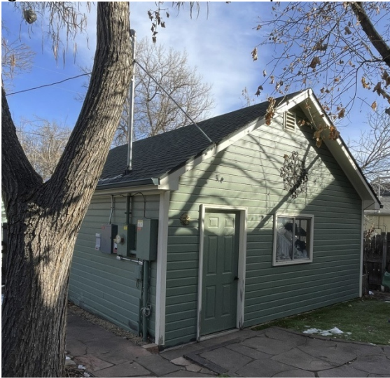
Electrical masthead and garage subpanel
