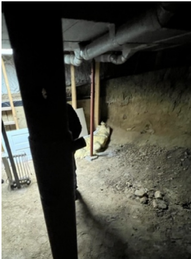
Figure 9: Improperly installed steel pin (Foreground) Over-extended post cap (Background)
