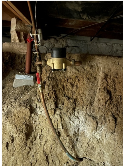
Domestic water tap and meter
