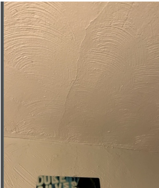
Figure 11: Painted over Ceiling Crack
