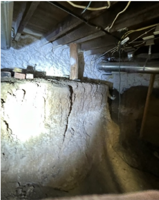
Figure 7: Precarious Beam Support
