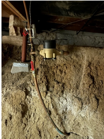
Domestic water tap and meter
