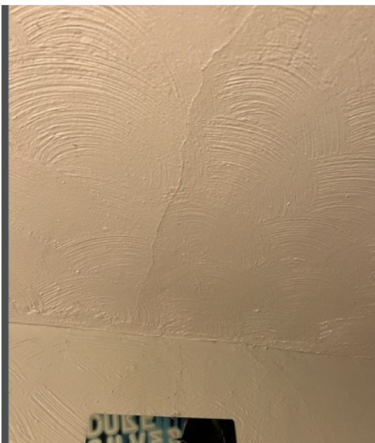
Figure 11: Painted over Ceiling Crack
