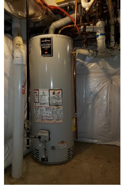
Water heater, supply, and waste lines in the basement.
