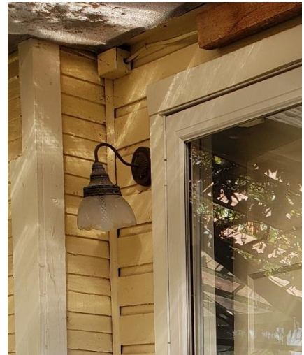
Wall sconce at the east addition.
