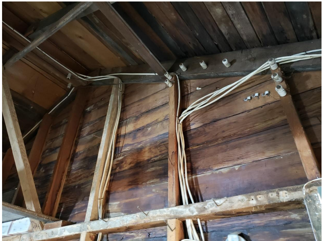
Romex wiring next to abandoned knob-and-tube wiring in the garage.
