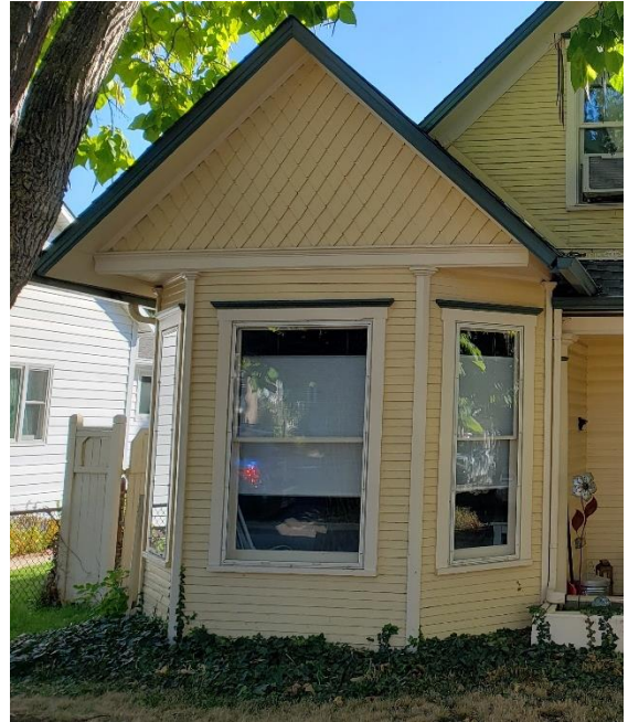
Ground covers growing on the house and the foundation.
