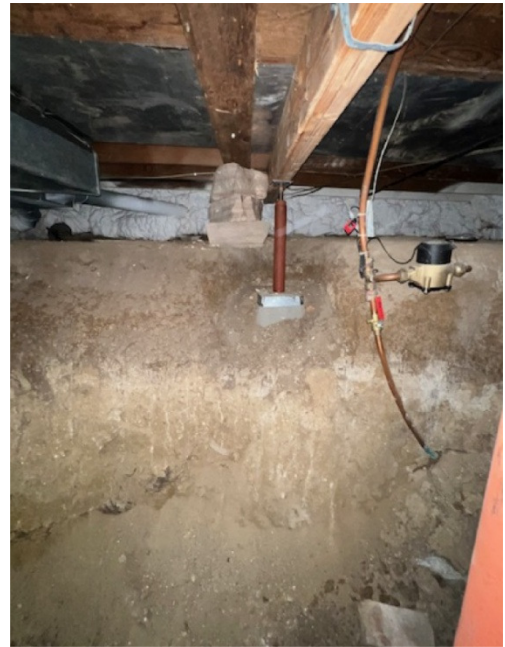
Figure 8: Supports near sloughing soil
