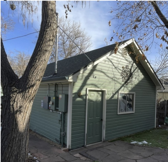
Electrical masthead and garage subpanel
