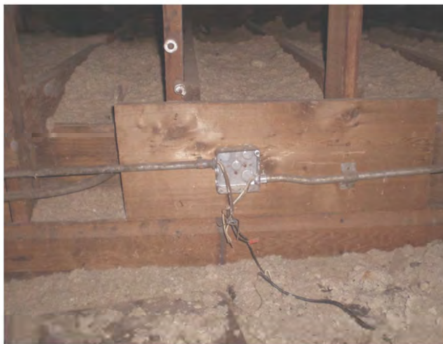
Electrical wiring and remainder of previous ceramic electrical system
