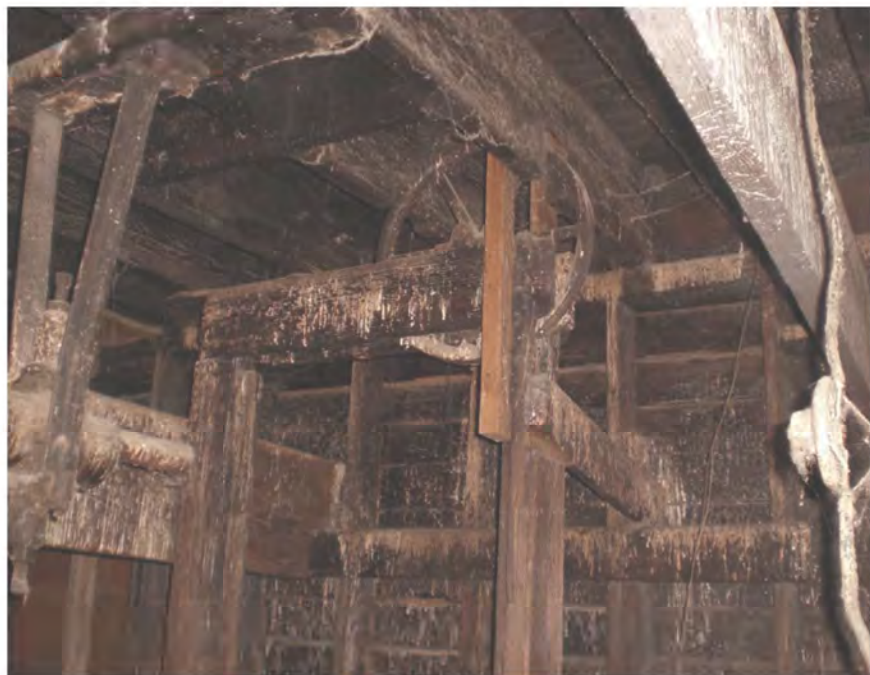
Fourth Floor - Equipment and Sixth Floor Structure with char damage and bird guano
