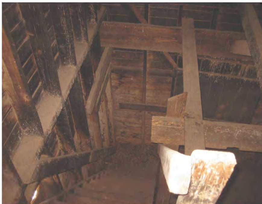
Section 3: Sixth floor exterior wall along grid 3 and grid A; unbraced wall hinge at break in studs
