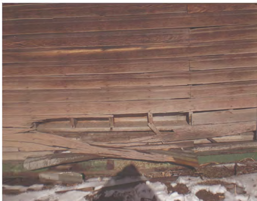
Section 5 - siding deteriorated at grade level of south elevation.
