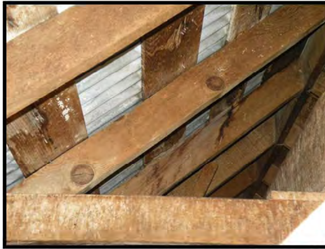
Figure 6. Large knots on a roof rafter above the Grain Bins (Section 4) that limit the structural grade.
