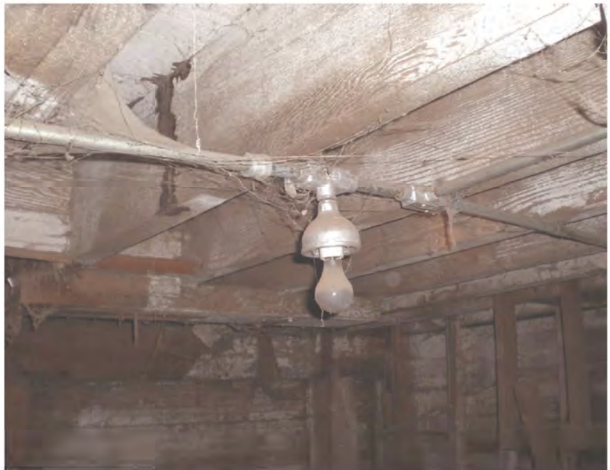
Light fixture and wiring in the basement
