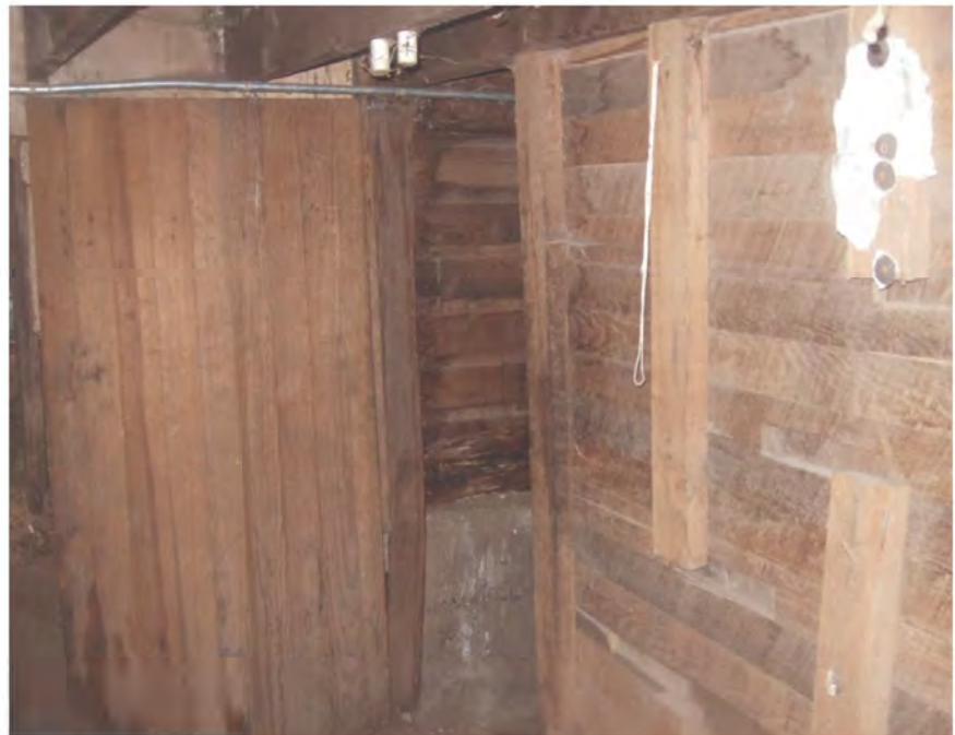
Door 3 propped open
