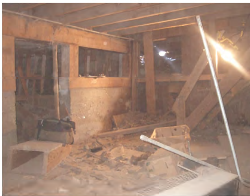
Section 2: Foundation wall along grid 3; basement stair, wall sheathing deterioration along grid Z
