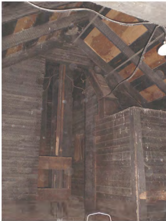
Second Floor - Char damaged on walls and grain bin on south side of the room
