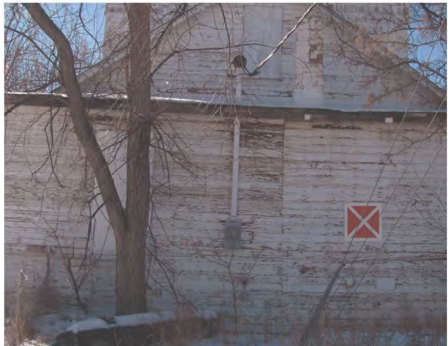
Weatherhead and electrical meter on the north side of the building
