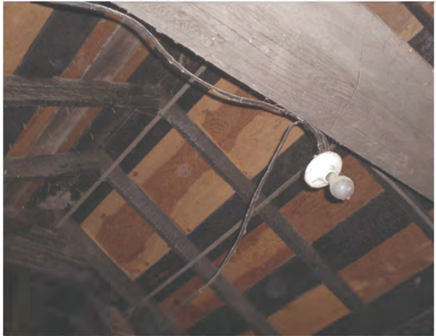
Wiring leading to the light fixture on the second floor and continuing on to the third floor
