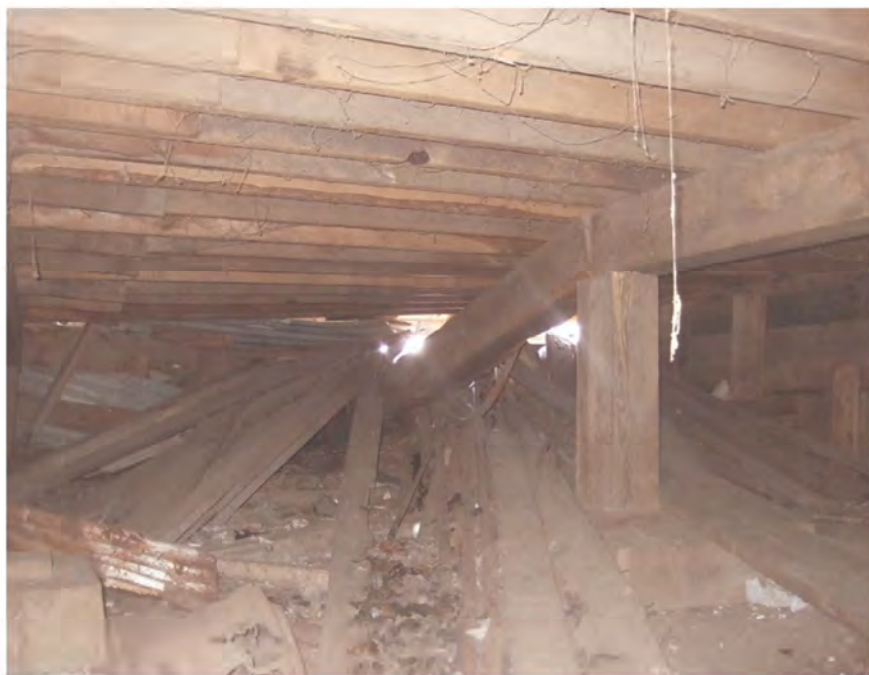
Section 5: Failed foundation wall along grid 6
