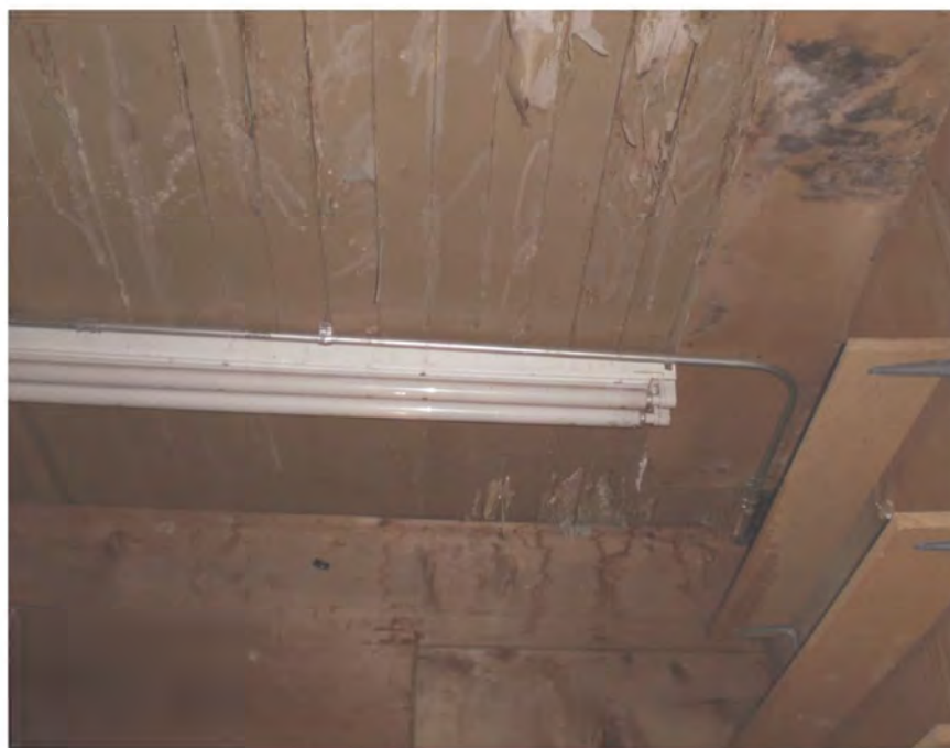
First Floor - Office ceiling damage
