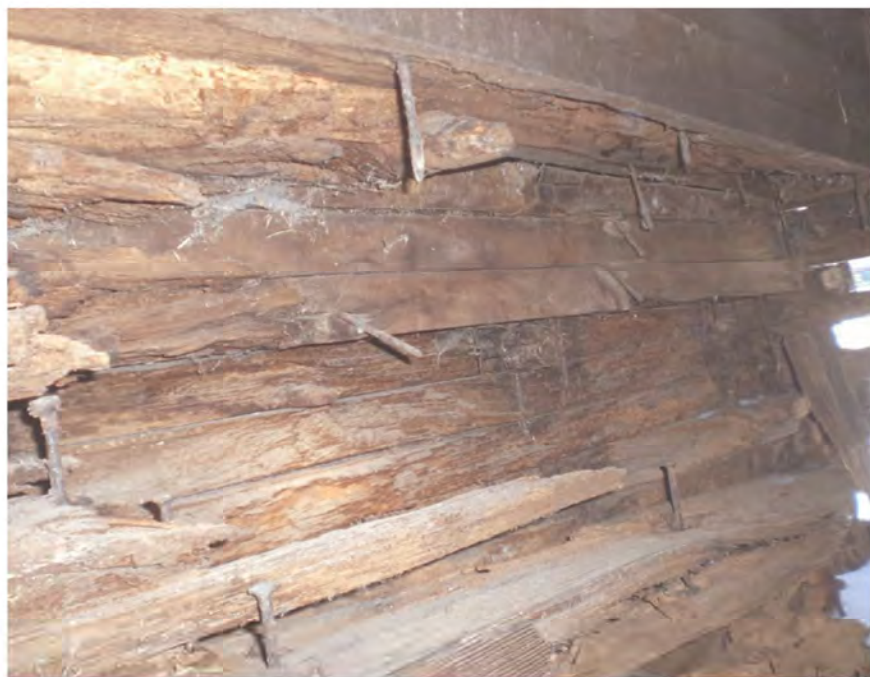
Section 4: Bin 5 wall detail view of deterioration, plank plies, and nails
