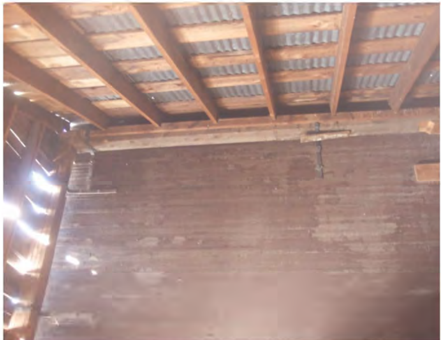
Section 5: Roof ledger along grid 5 and underperforming anchors into stacked-plank wall
