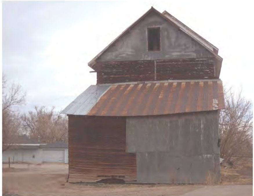
Section 5: Settled stud wall and roof framing along grid 6
