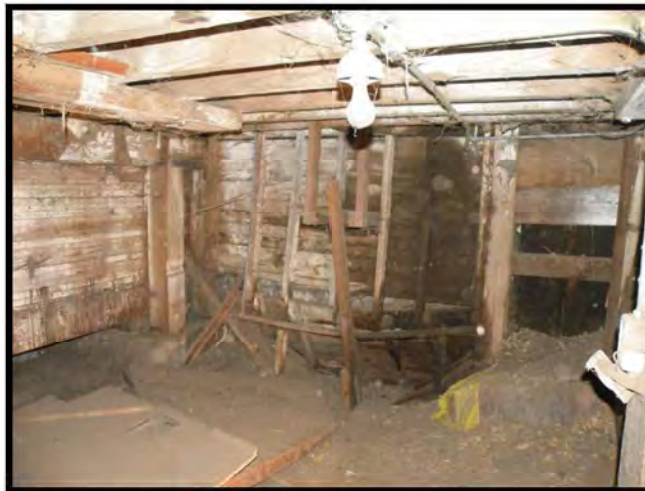
Figure 4. Interior view of the west basement wall of Section 3, Level 0, which has collapsed due to deterioration caused by wood decay fungi.
