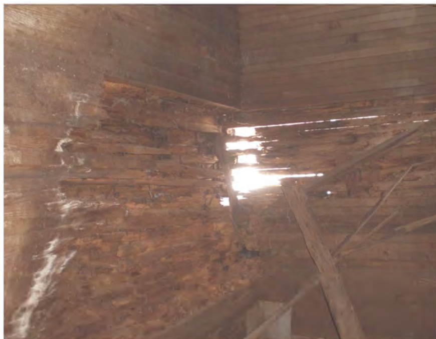
Section 4: Southwest corner of Bin 5 wall deterioration near exterior grade elevation
