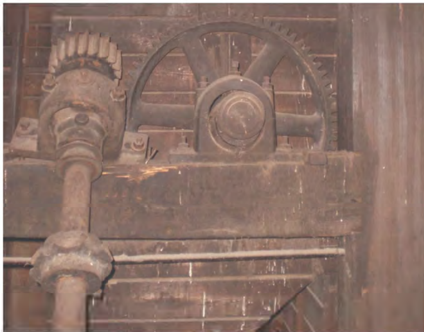
Elements of the conveying system on the sixth floor
