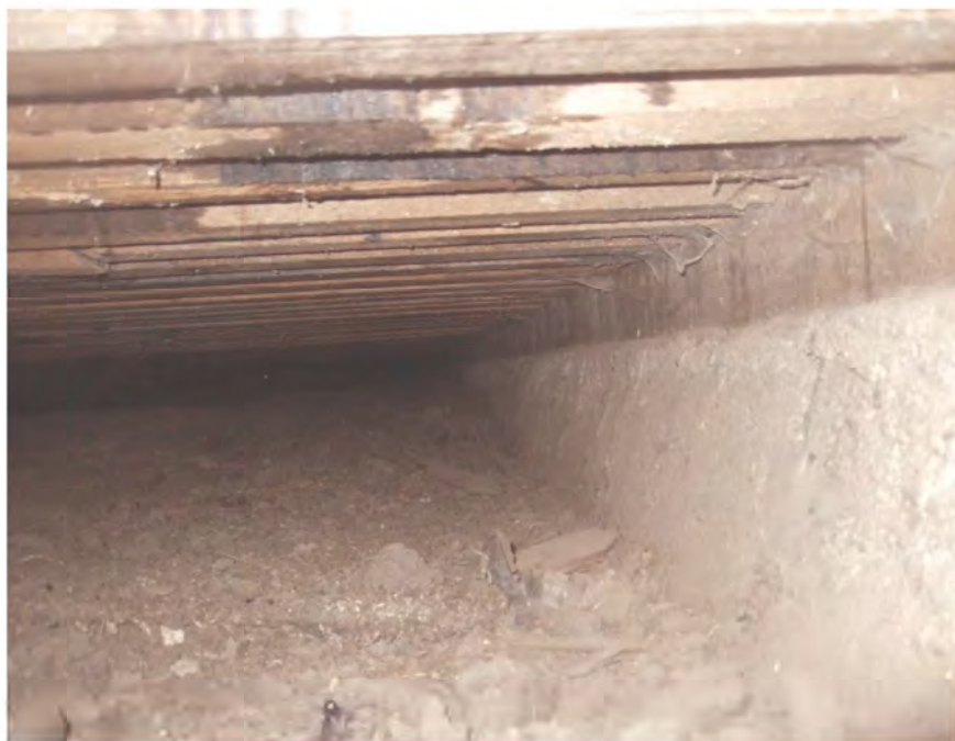
Section 4: Underside of Bin 4 floor along grid Z
