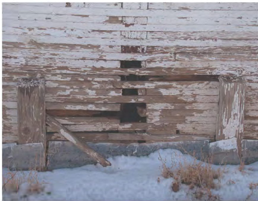
Section 4 - deteriorated cribbing at grade level
