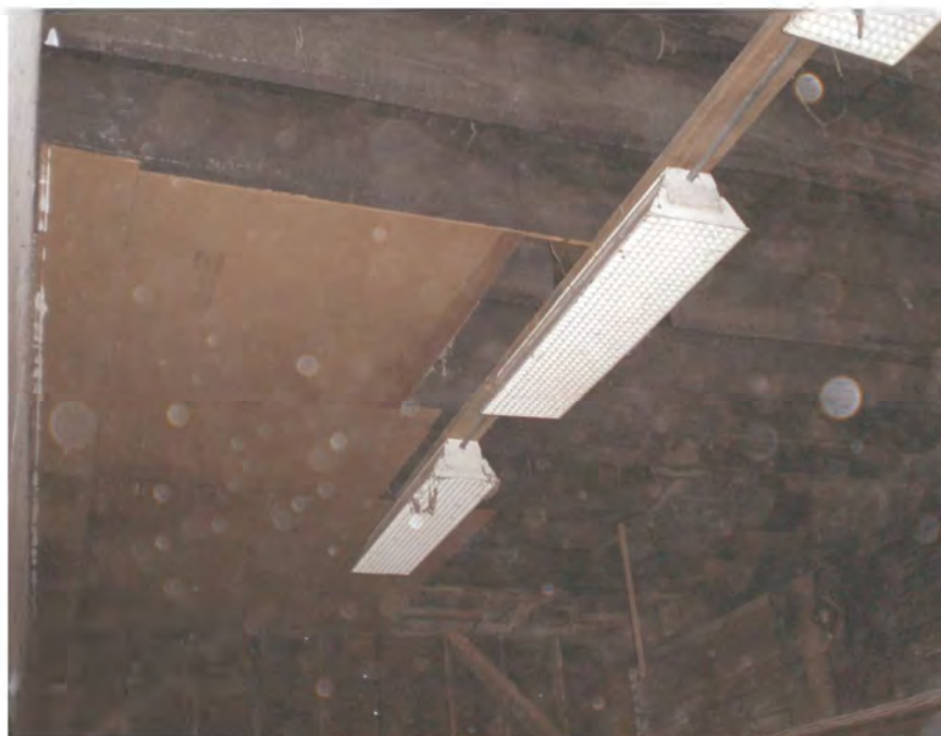
Fluorescent light fixtures in Tower Level 1
