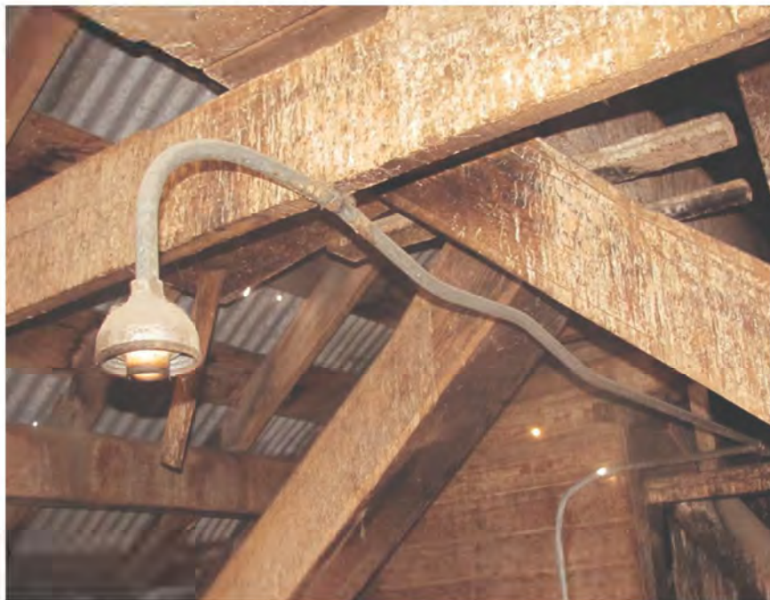
Light fixture over the platform over the grain bins
