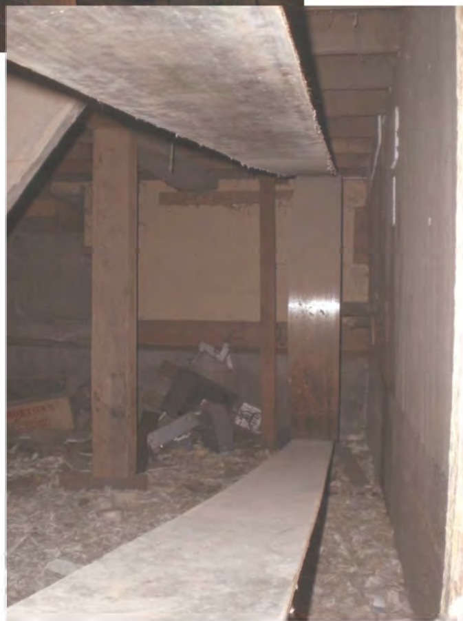
Large pulley and belt in the Machine Room in the basement
