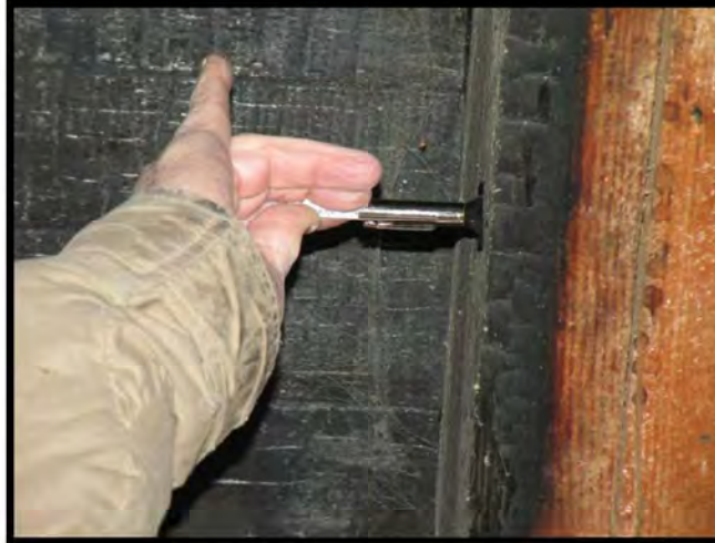
Figure 7. Measuring the depth of char on a joist with a char depth gauge. Note the alligatoring on the floor sheathing above the joist.
