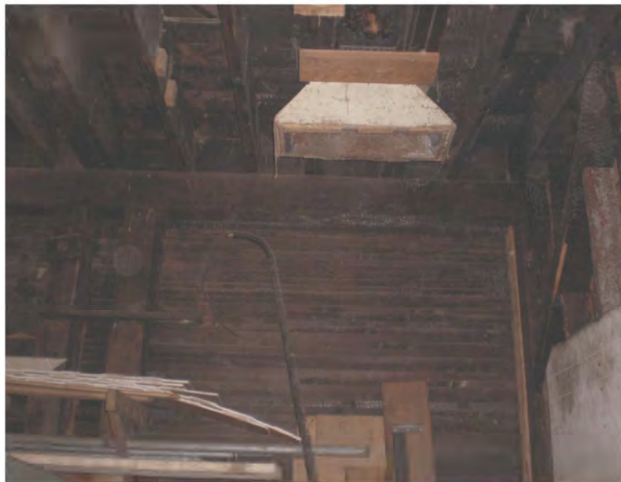
First Floor - Tower Level 1 chute on ceiling and char damage on walls and ceiling
