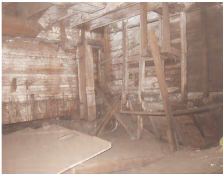
Section 3: Foundation wall along grid Z near grid 3; wall failure along grid Z
