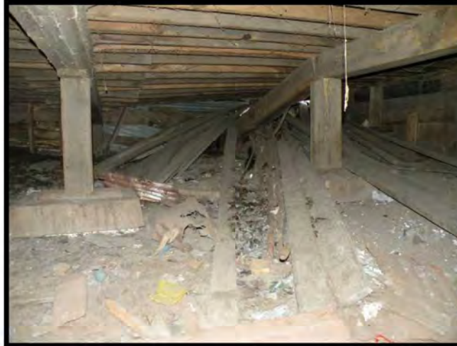
Figure 5. Interior (crawl-space) view of the south foundation of Section 5 with collapsed elements.
