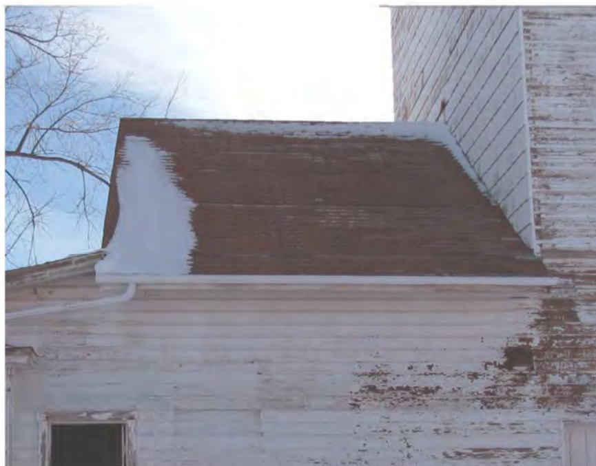
Gutter, downspout and deteriorated asphalt roofing on Section 2
