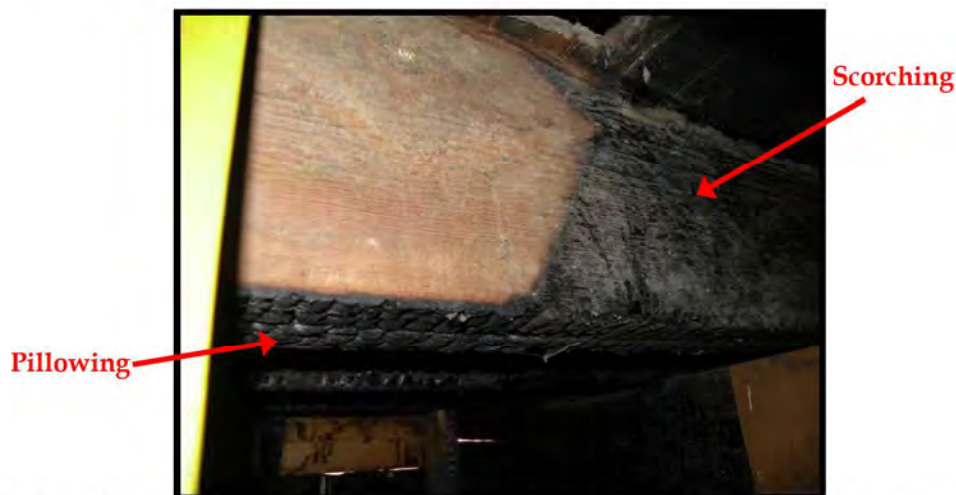
Figure 8. Pillowing and scorching on the same joist, Section 3, Level 1. Areas of undamaged wood are visible where charred elements have been removed.
