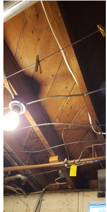
Floor framing bears on a 2x sill plate with an uninsulated rim joist.
