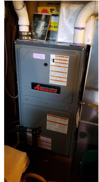
Gas furnace located in the basement.
