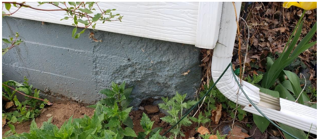
Foundation deterioration at the northeast corner. The added downspout extension appears to have remedied the issue.
