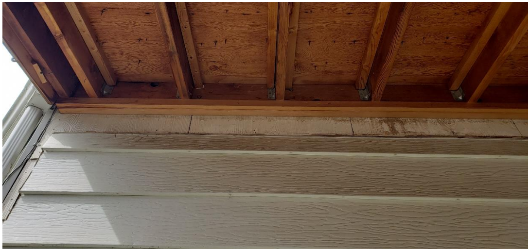
Asbestos siding is visible below the new patio roof.
