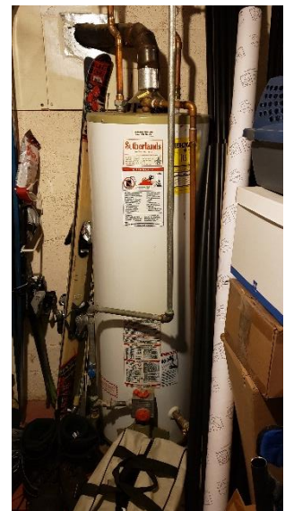
Gas water heater located in the crawlspace.
