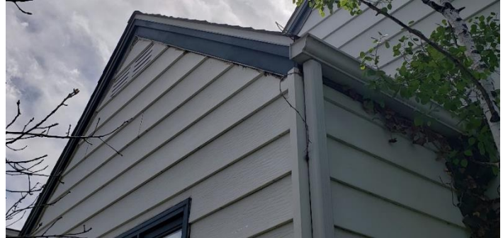
Front gable showing painted wood fascia that is partially covered by the metal drip edge and gutters.
