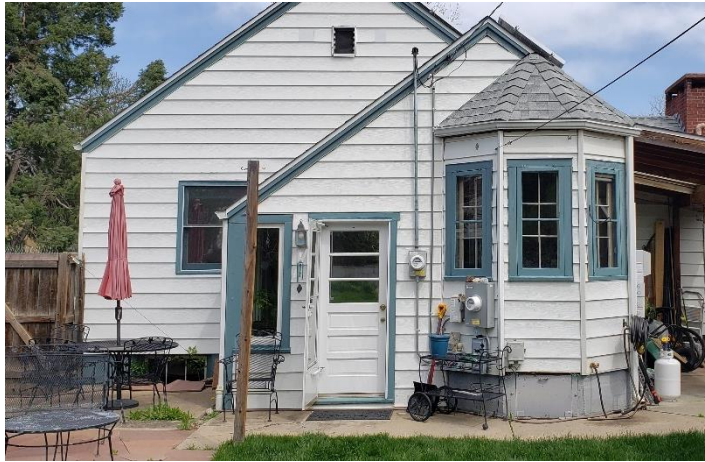
The foundation is exposed in most areas except for at the rear entry.
